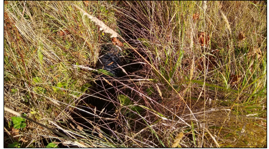
Photo 10. A corrugated plastic pipe drains to the upper end of the ditch on the adjacent property. The pipe may drain from the base of the retaining wall upslope of the residence on that property.
