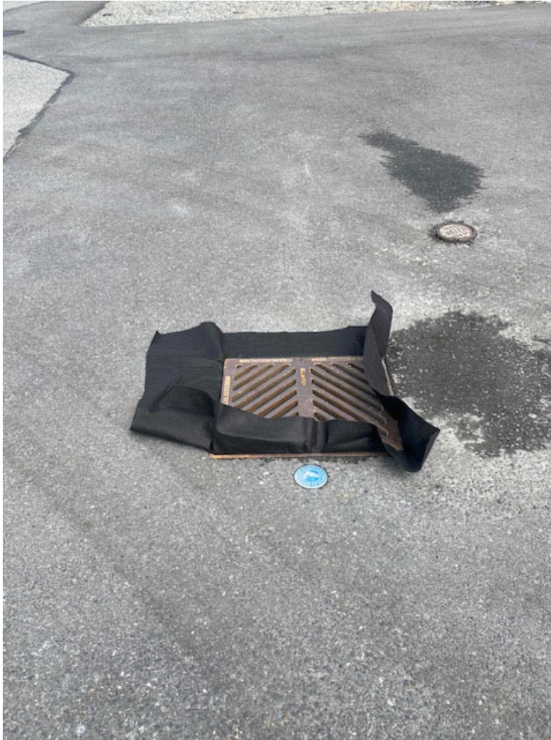
Photograph 1 Typical Storm Inlet Protection Installed
