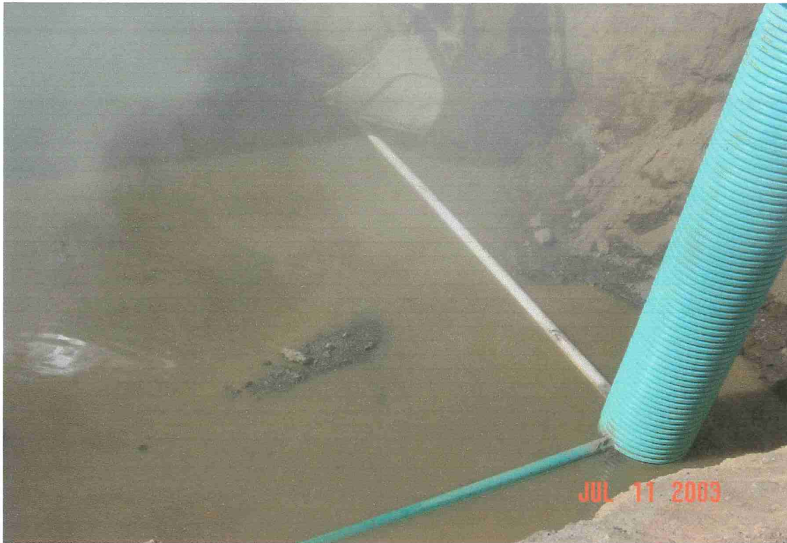
Collection piping-water level & piping is approximately 12' below grade
