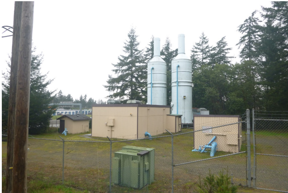
Groundwater treatment facility at wells H1 and H2.
