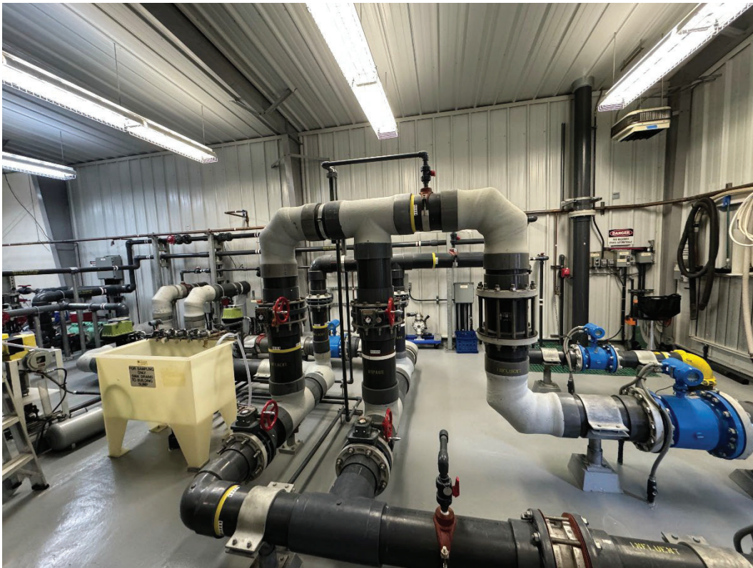
Piping inside groundwater extraction and treatment facility
