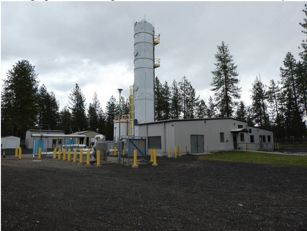
Groundwater extraction and treatment tower and building
