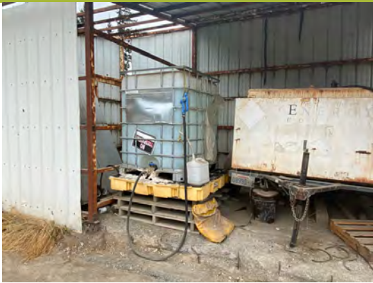
Photograph #19: Diesel exhaust fluid AST.
