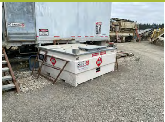
Photograph #36: Diesel AST
