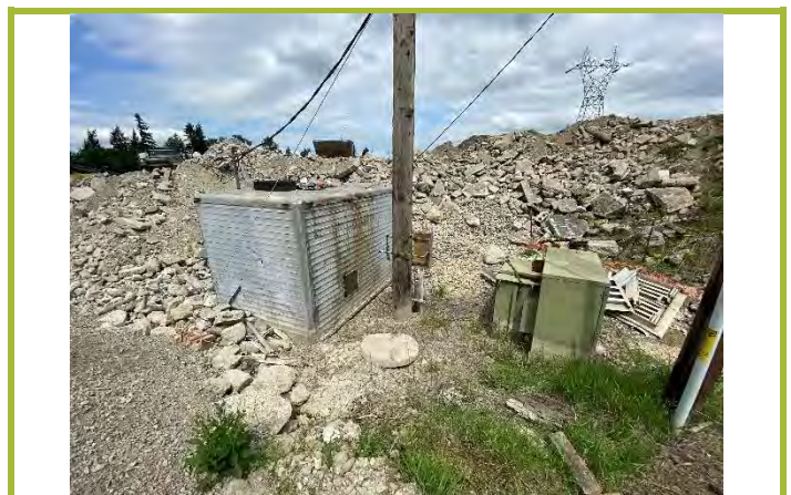
Photograph #18: On-site transformer in southeast portion of the Subject Property.
