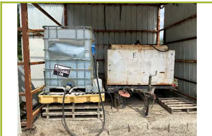
Photograph #23: Diesel exhaust fluid AST.
