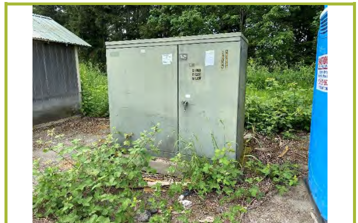
Photograph #30: On-site pad-mounted transformer on the northwest portion of the Subject Property.
