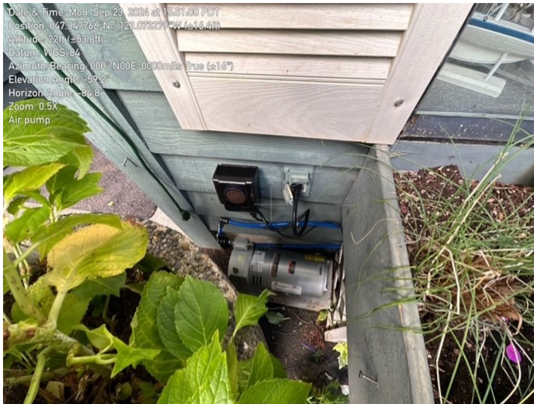
Photograph 4.6. View of the rotary vane compressor used to pump air into the groundwater. The compressor was on a timer for nighttime operation.
