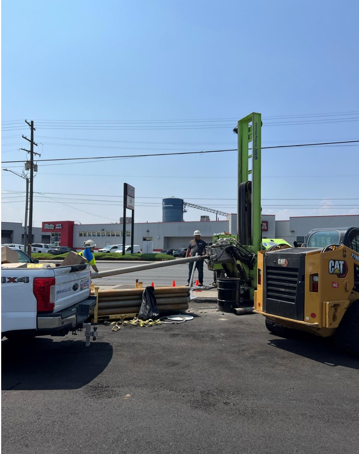
Photograph 5 – Terra sonic drilling rig set-up to advance boring MW9 on May 19, 2023 (facing west).
