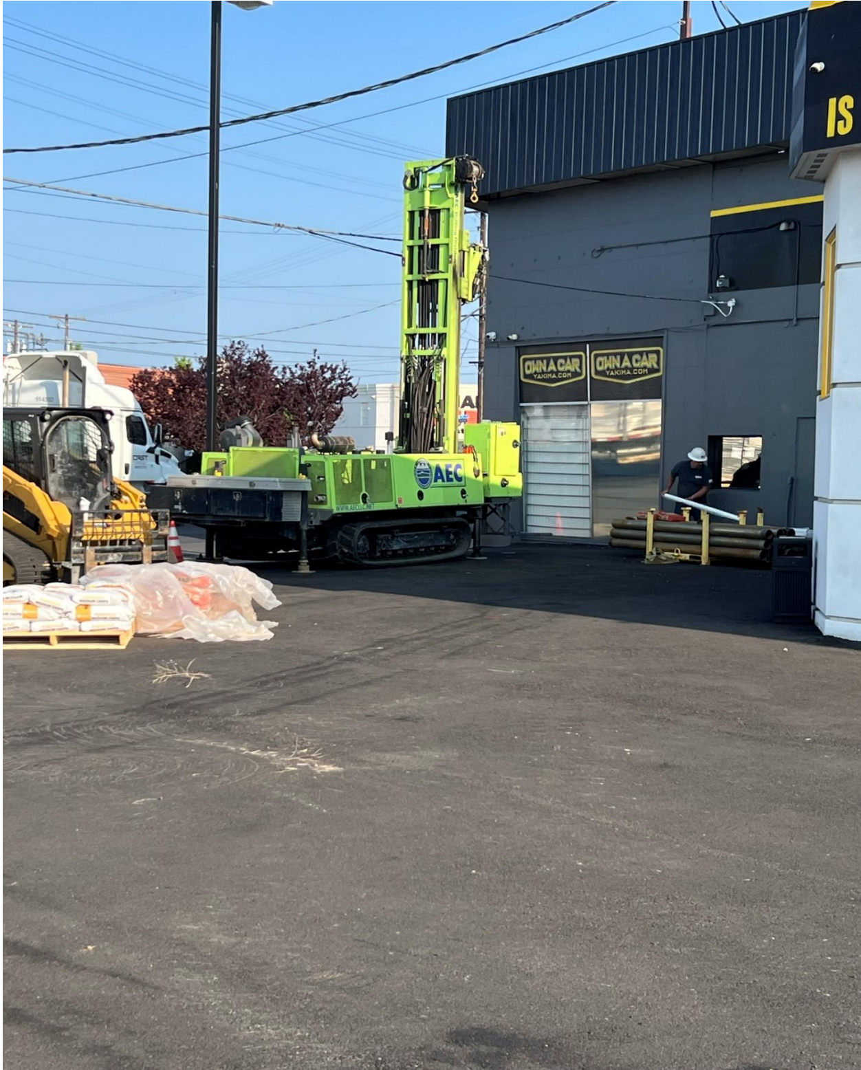
Photograph 1 – Terra sonic drilling rig set-up to advance boring MW7 on May 19, 2023 (facing NW).
