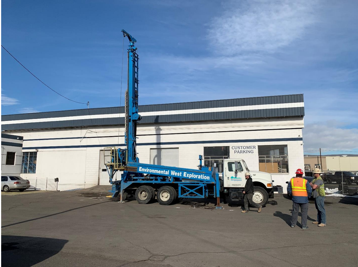
Photograph 7 – View of sonic drill rig prepared to begin drilling at soil boring SB1 on Tuesday, February 1, 2022 (facing north).
