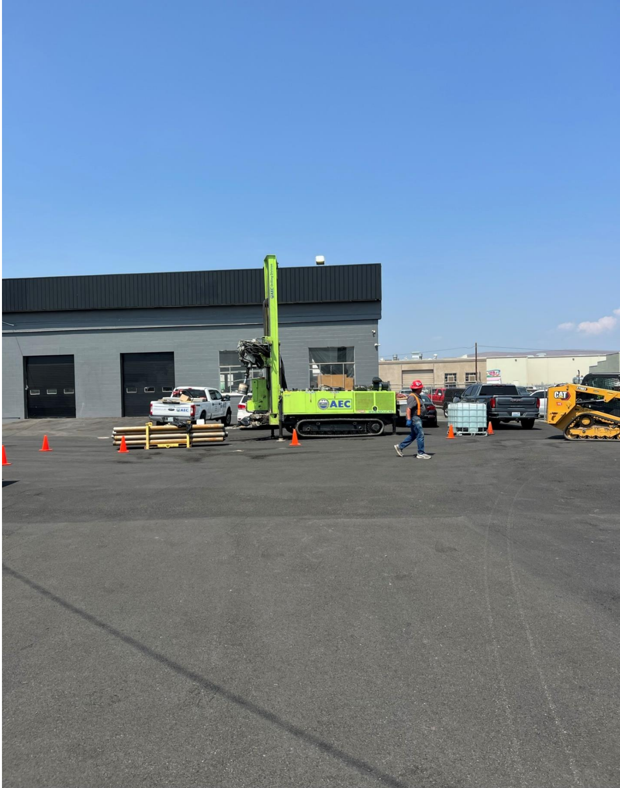
Photograph 6 – Terra sonic drilling rig set-up to advance boring MW3A on May 19, 2023 (facing north).
