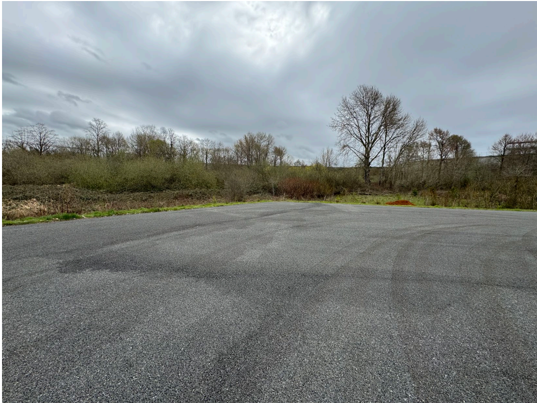
Photograph D4. Stations DMCA 06, 07, and 08. Previously noted area of potential material loss is stable in DMCA 06 and 07.
