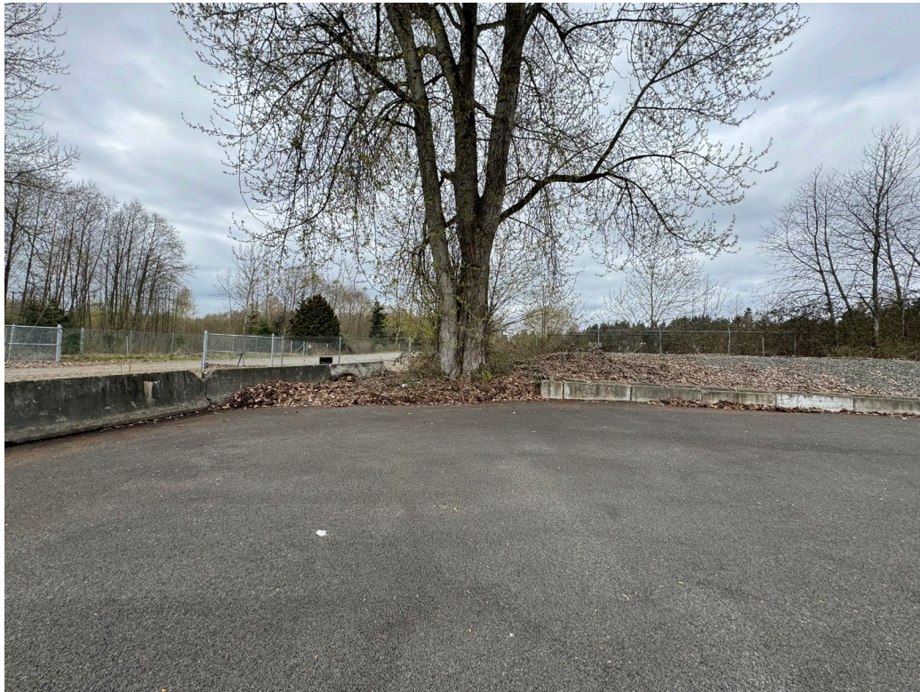
Photograph D5. Stations DMCA 09. Presence of debris on barrier surface.
