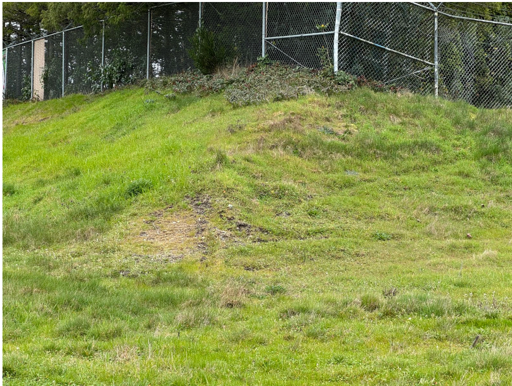
Photograph L4. Stations LLA 11, LLA 12, and LLA 13. Loss of barrier material.
