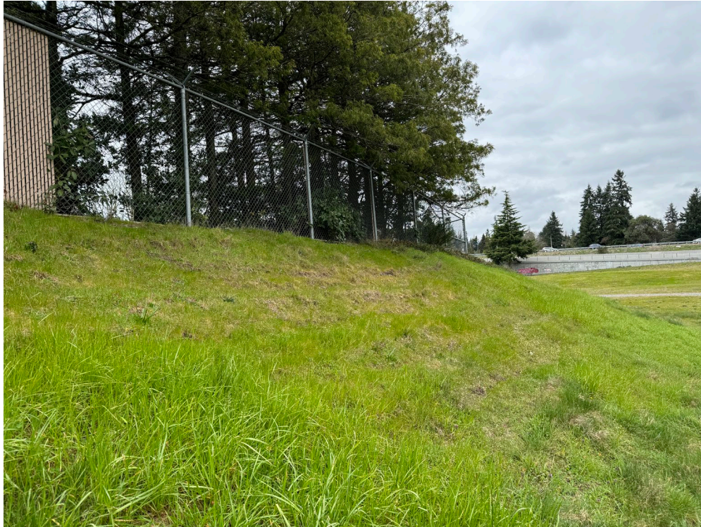
Photograph L5. Station LLA 12. Loss of barrier material.
