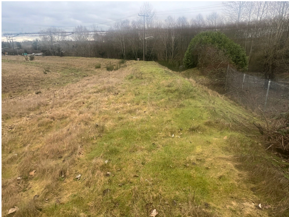
Photograph 4. Reseeded area near Station LLA 14 at the Lora Lake Apartments Parcel looking east. The area previously showed signs of loss of barrier material.
