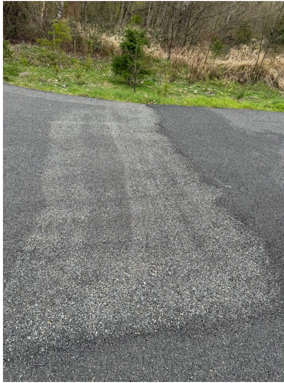
Photograph D3. Previously noted area of potential material loss between DMCA 04 and DMCA 05 is stable.
