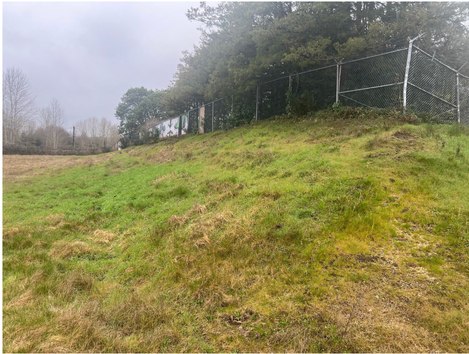
Photograph 1. Reseeded slope near Stations LLA 12 and LLA 13 at the Lora Lake Apartments Parcel looking southwest. The area previously showed minor loss of barrier material.
