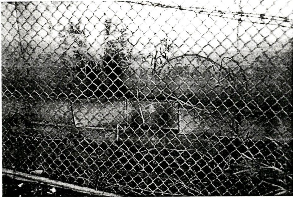
Cracked Berm Blocks
