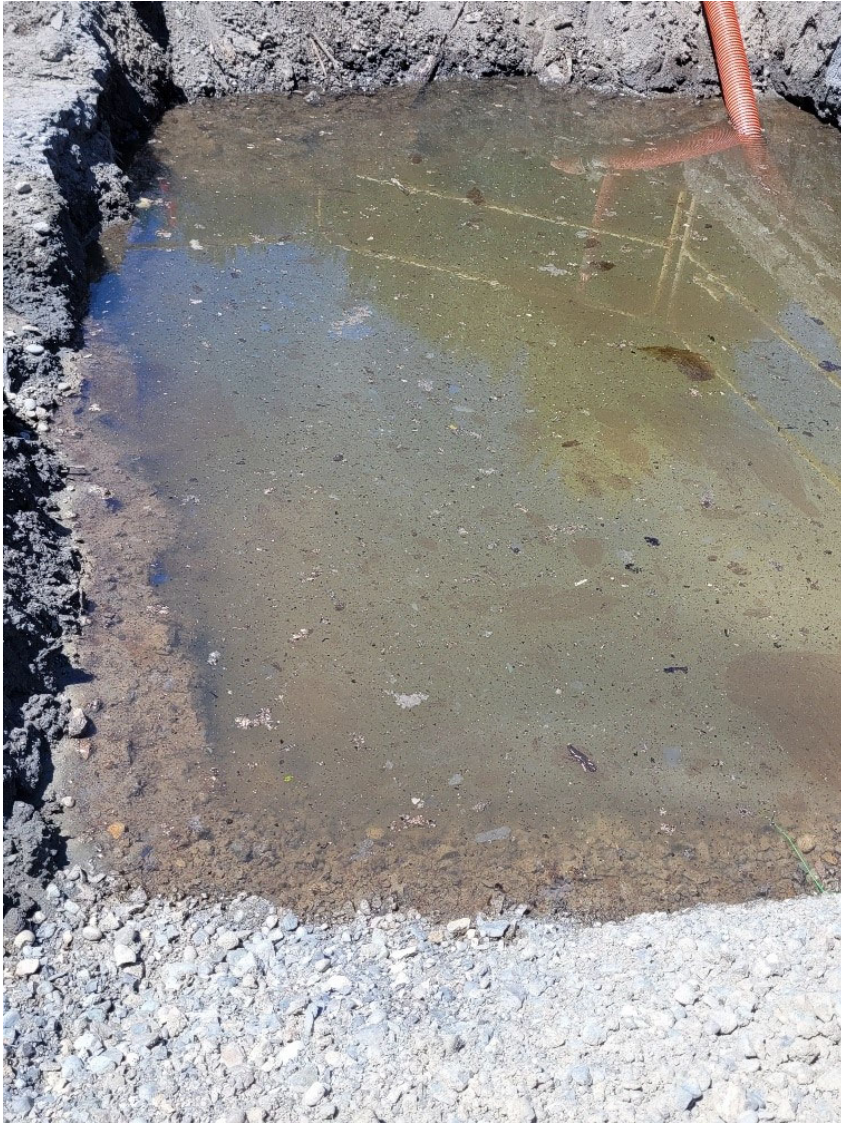
Figure 2 Photo of excavation pit with visible blobs of oil present, the surface is about 10 ft by 10 ft and approximately 15 blobs of oil were noted on the surface. This photo was taken 4 days after the excavation was opened.
