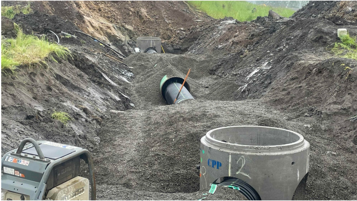
Installation of 48-inch manholes at Stations D0+05 and C0+12, 24-inch CPE pipe, and 30-inch steel pipe casing
