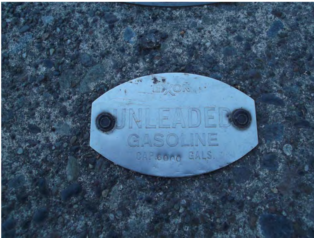
Photograph 3 – View of tag, with Exxon logo, installed adjacent to the fill port of the northeastern-most fuel storage UST, indicating a 6,000 gallon capacity unleaded gasoline tank. No other UST fill ports had similar tags.
