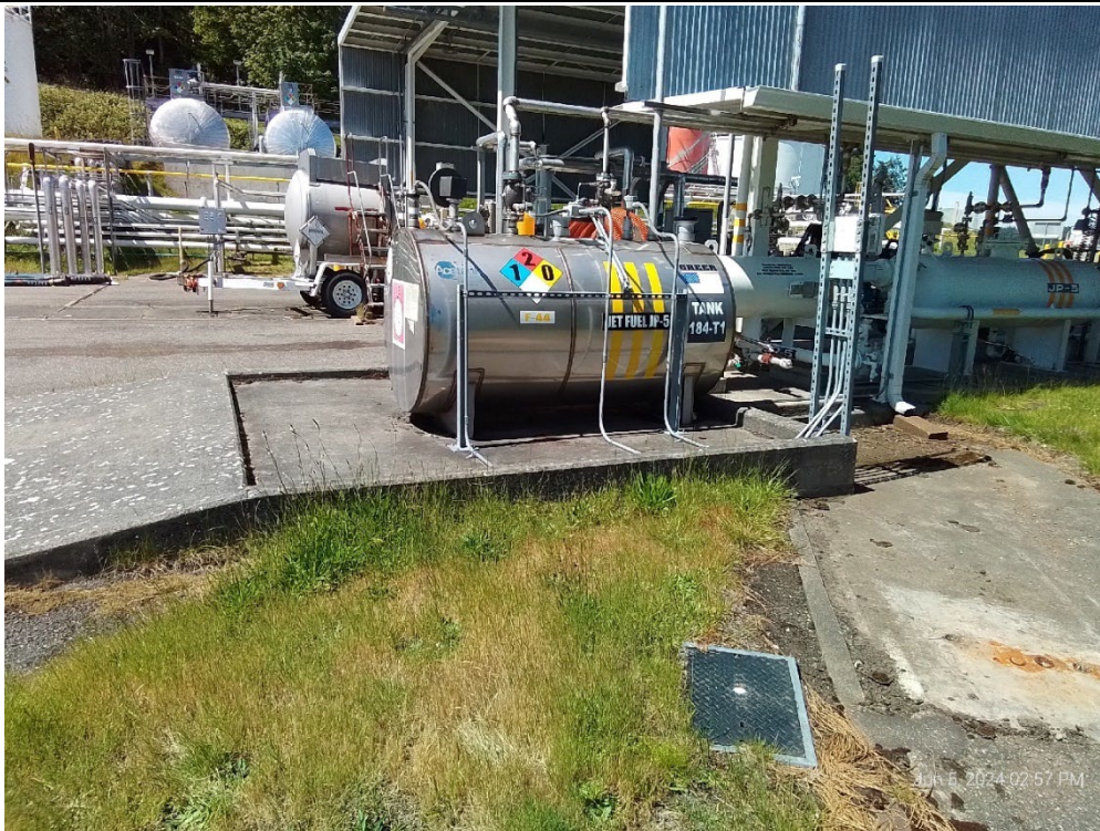
Photograph 12 Fuel related waste storage containers (under canopy), facing northwest.
