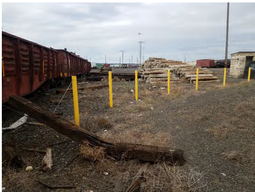
Photograph 6 – damage to southwestern fence corner. 6/28/2018
