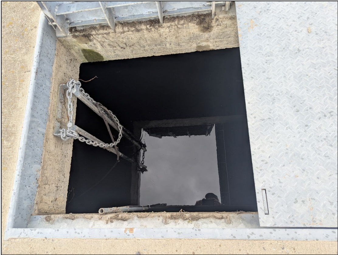
Water filling in West Pump Vault indicating need for repairs
