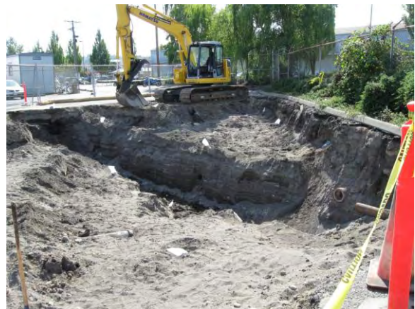
Photo 6D: Excavation – all BRPH-impacted material removed, north end of excavation area looking southwest.
