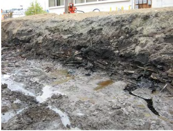
Photo 15B: BRPH-like free product draining from north sidewall adjacent to south side of East 19 th Street UST looking northwest.
