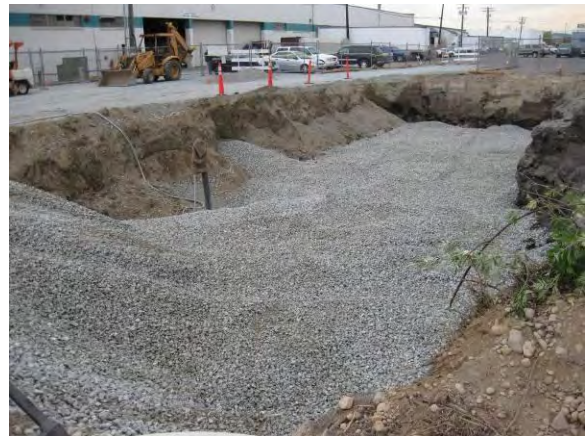
Photo 63B: Excavation backfilling – southwest corner of Phoenix excavation area looking northeast. 2-inch ballast in place.
