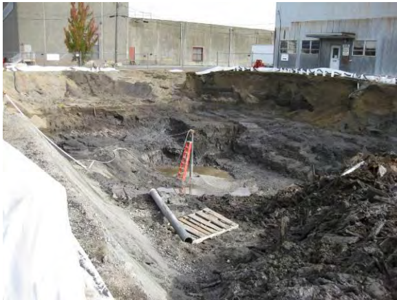
Photo 23C: Excavation – deepest portion of area approximately 19 feet below grade surface at center of photo. North end of excavation area looking northeast.
