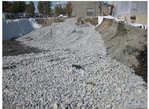
Photo 42C: Excavation backfilling – spreading quarry spalls across bottom of north half of excavation area looking north.
