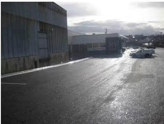
Photo 54C: Post remediation – new asphalt parking lot for SuperValu, north end of excavation area looking southeast.
