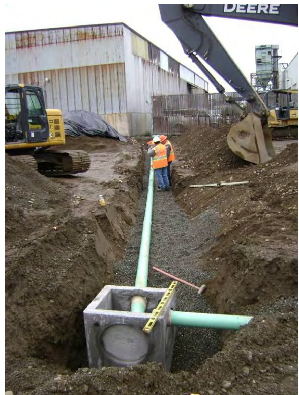
Photo 36C: Utility reconstruction – storm sewer lateral catch basin for south end of SuperValu parking lot looking northeast.
