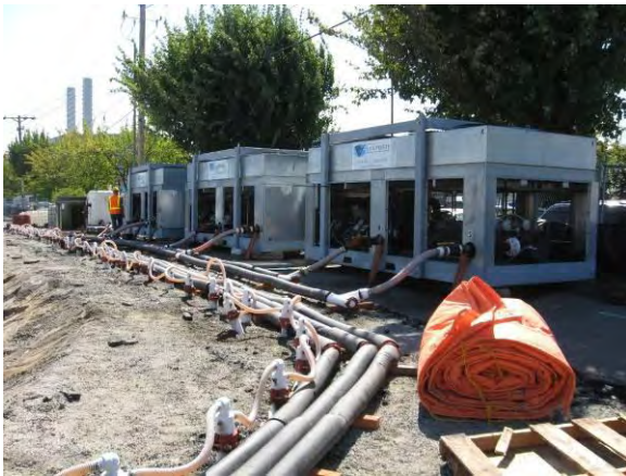
Photo 8C: Freeze wall chillers – north end of west side of excavation area. Freeze wall manifolding wrapped with foam insulation.
