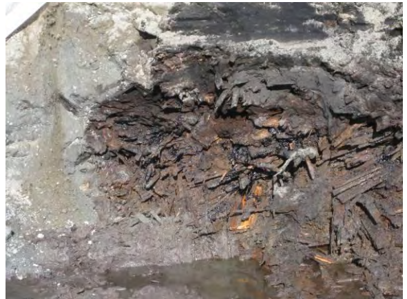
Photo 20C: East sidewall – northern extent of wood waste exposed in sidewall with BRPH free product. Bank run backfill to left of wood waste from previous excavation under SuperValu building footprint.
