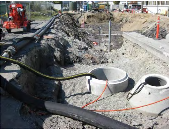
Photo 46B: Utility reconstruction – new sanitary sewer manhole at southeast corner of Area B with bypass system.
