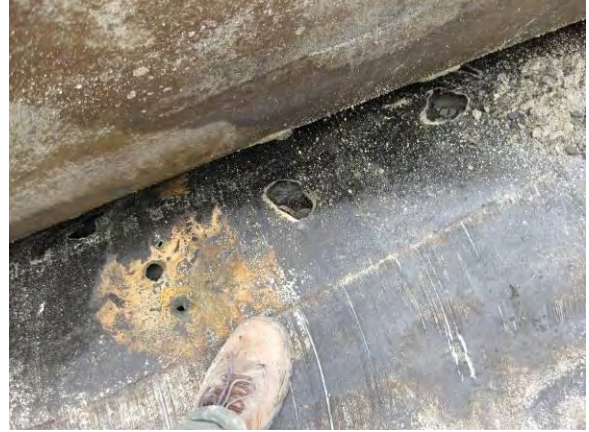
Photo 28B: East 19 th Street UST - Note: observed fist-sized holes corroded through side of UST.
