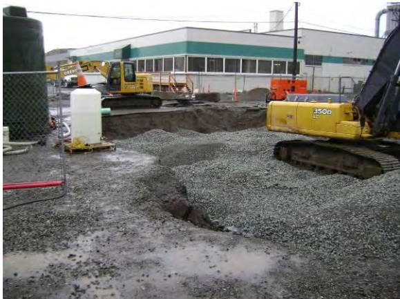
Photo 68B: Excavation backfilling – excavation area west of Phoenix lay down yard looking northeast.
