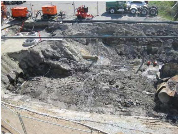
Photo 34B: Excavation area – east end looking south. Sewer and storm bypass pumps in upper left of photo.
