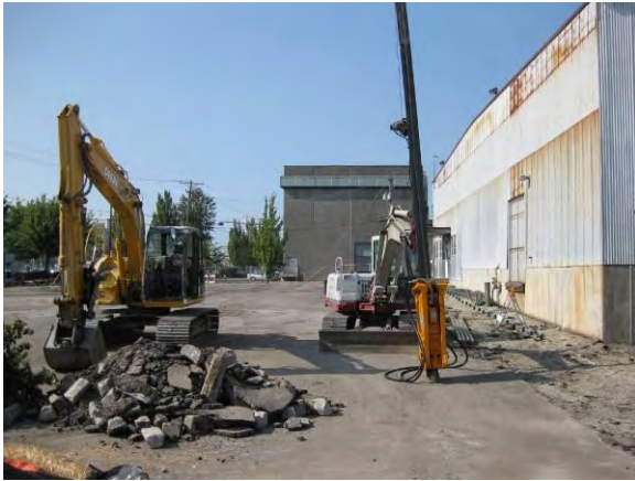
Photo 6C: Freeze wall installation – rotohammer attached to miniexcavator used to drive freeze pipes.
