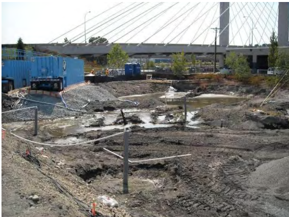
Photo 11A: Excavation dewatering – water treatment system includes blue tanks in upper left and center. South end of excavation area looking southwest.
