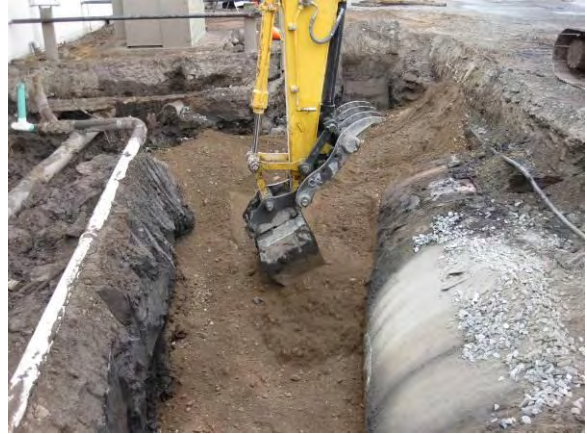
Photo 56B: Excavation backfilling – north side of East 19 th Street UST within Safe Dig Area looking east.
