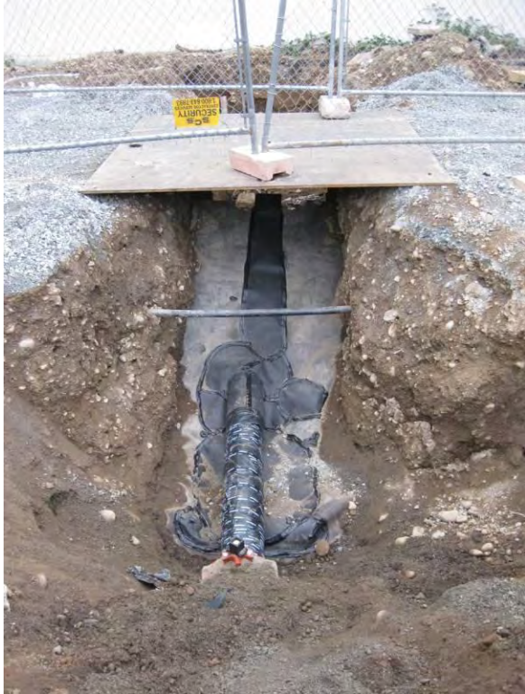
Photo 55B: Utility reconstruction – fire service line for Tacoma Fixtures with welded penetration through Area B HDPE liner looking north.
