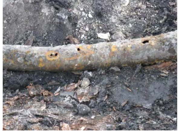
Photo 40C: BNSF Oil Pipeline with holes and corrosion at north end of excavation area.
