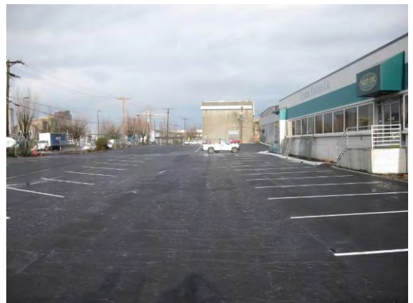
Photo 55C: Post Remediation – new asphalt parking lot for Tacoma Fixtures, south end of excavation area looking north.
