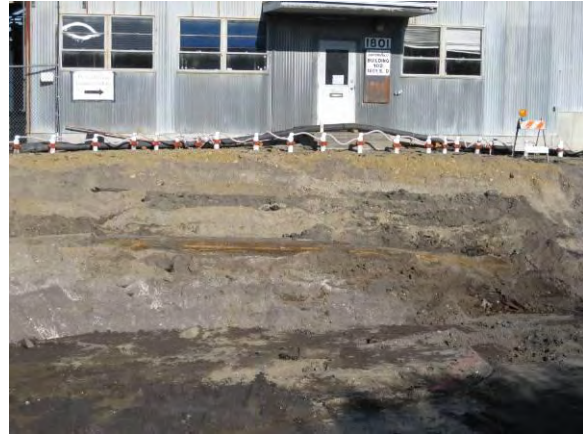
Photo 14C: BNSF Oil Pipeline – rust colored alignment crossing center of photo. Looking east toward SuperValu building.
