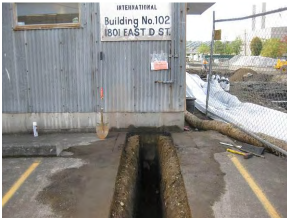
Photo 31C: Utility reconstruction – natural gas service trench to northwest corner of SuperValu building.
