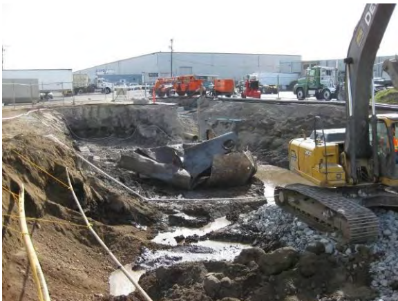
Photo 31B: East 19 th Street UST - removed UST placed in excavation looking southeast.
