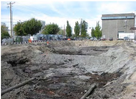
Photo 15C: Segments of BNSF Oil Pipeline lying in excavation. Natural gas service crossing excavation from left to right. East side of excavation area looking north.
