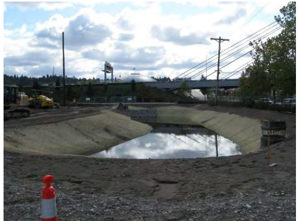
Photo 28A: Pond rebuilding – hydroseed placed around ponds for erosion control. North end of excavation area looking south.
