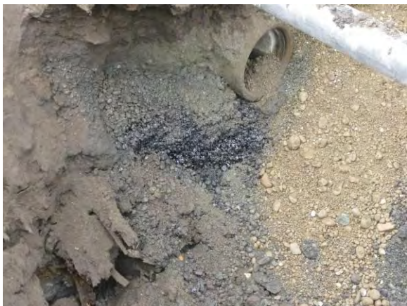
Photo 36B: West sidewall with 12-inch sanitary sewer line exposed. Pea gravel in sewer trench saturated with BRPH-like free product.
