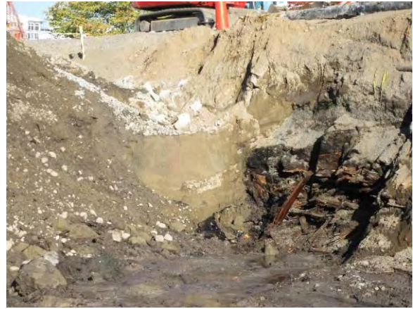
Photo 18B: Excavation area – northwest corner looking northwest. Note: observed 2004 Interim Action CDF and BRPH-like free product draining from wood waste at center of photo.
