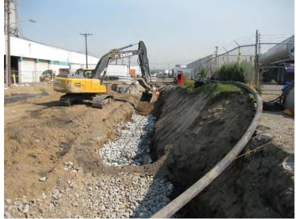
Photo 61B: Excavation backfilling – sanitary sewer subgrade reconstruction along south side of Area B looking east.
