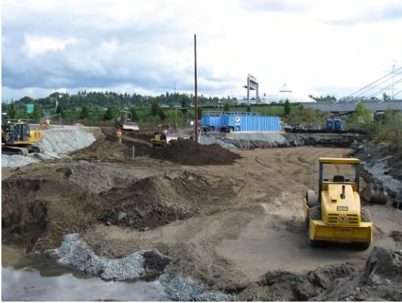
Photo 21A: Excavation backfilling – placing bank run fill across excavation base. North end of excavation area looking south.
