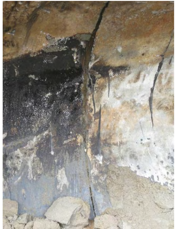
Photo 30B: East 19 th Street UST - Note: observed failed weld seen inside UST.
