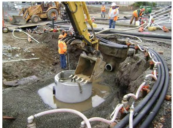
Photo 32C: Utility reconstruction – sanitary sewer manhole placement south end of excavation area looking southeast.
