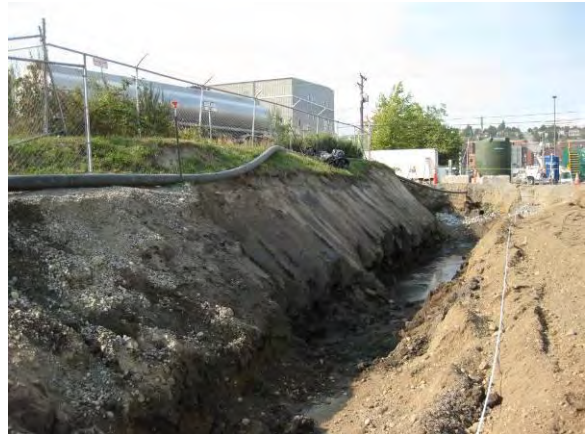
Photo 35B: Excavation area – south sidewall adjacent to the north side of Phoenix lay down yard. Trench represents East 19 th Street sanitary sewer alignment.
