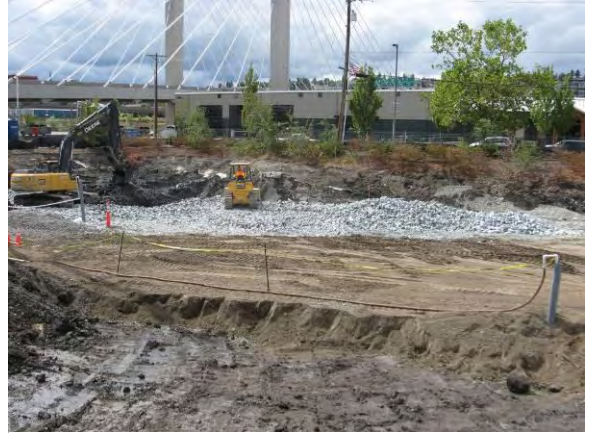
Photo 22A: Excavation backfilling – placing quarry spalls under south end of WSDOT ponds looking west.
