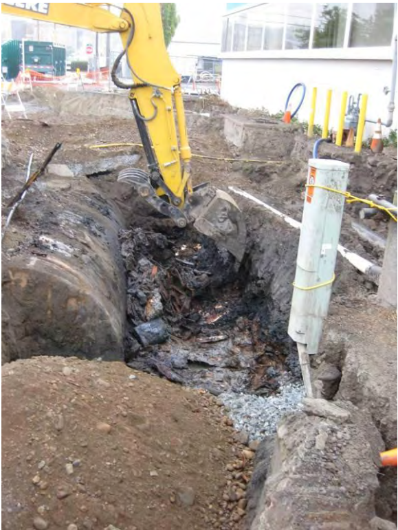
Photo 12B: East 19 th Street UST – excavating along north side of UST within Safe Dig Area looking west.
