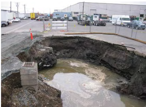
Photo 40B: Nichols area excavation – west end of excavation looking east with groundwater level after ½ day.
