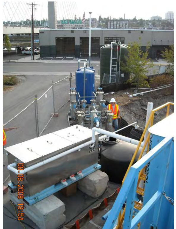
Photo 16A: Dewatering/treatment system looking west.
