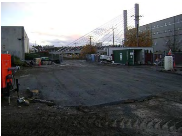
Photo 70B: Site grading – excavation area west of Phoenix lay down yard looking south.
