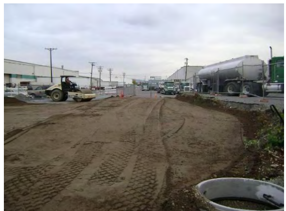
Photo 71B: Excavation backfilling – final lifts of bank run backfill for Phoenix excavation. West end of excavation looking east.
