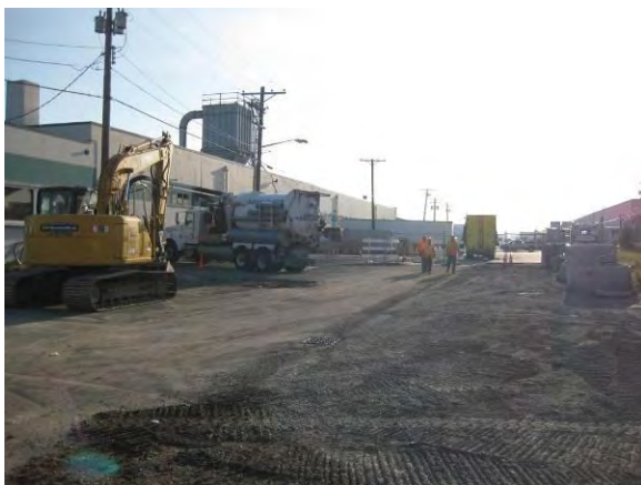
Photo 9B: Excavation area southwest corner looking northeast. Vactor truck working in Safe Dig Area.
