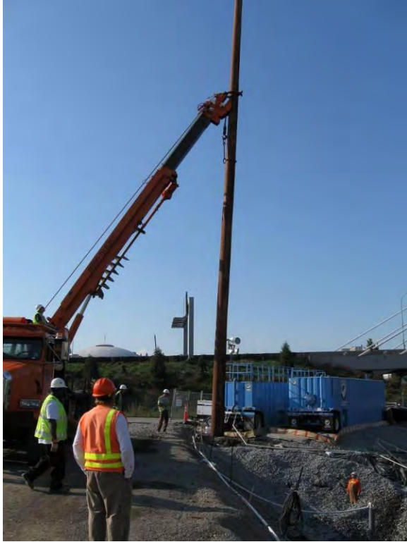
Photo 17A: Guy pole installation for power pole anchor from WSDOT pond area to the east of excavation area.
