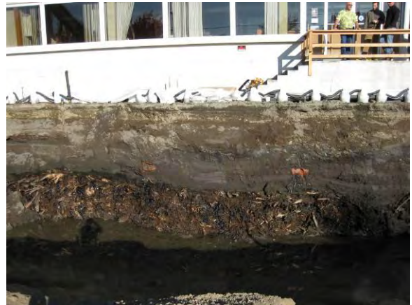
Photo 24C: Soil freeze wall – east sidewall in front of Tacoma Fixtures building. Wood waste overlain by soil fill.
