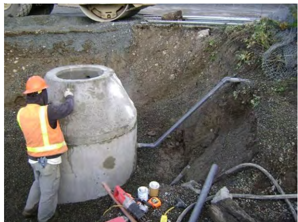
Photo 54B: Utility reconstruction – constructing the Phoenix Environmental sanitary sewer discharge lateral manhole.
