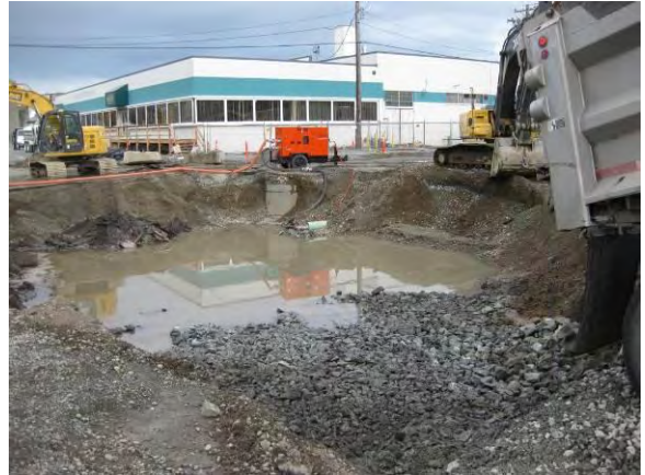
Photo 67B: Excavation backfilling – excavation area west of Phoenix lay down yard looking northeast.
