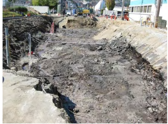
Photo 22B: Excavation area - east end looking west. Note: native tidal deposits across base of excavation and wood waste exposed in north sidewall.
