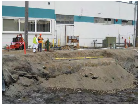
Photo 24B: East 19 th Street UST - marine chemist testing void space for explosive vapors.
