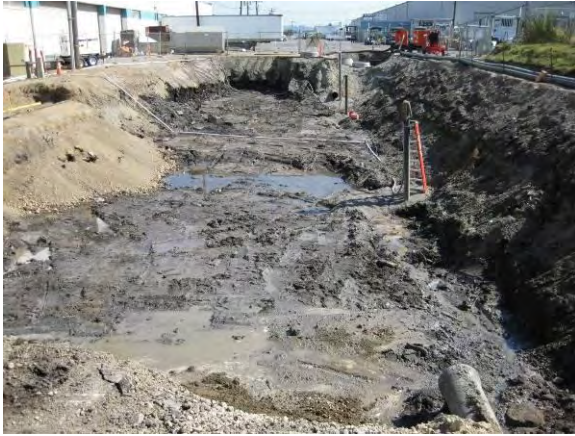
Photo 21B: Excavation area west end looking east. East 19 th Street UST exposed to the left.
