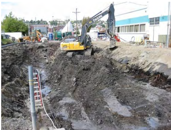
Photo 19B: Excavation area - east end looking west. Dewatering sump left side of photo.
