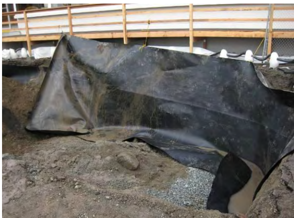
Photo 48C: HDPE liner – southeast corner of excavation area with additional HDPE liner placement.
