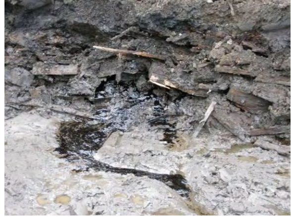
Photo 16B: BRPH-like free product draining from sidewall of excavation, adjacent to south side of East 19 th Street UST looking northwest.
