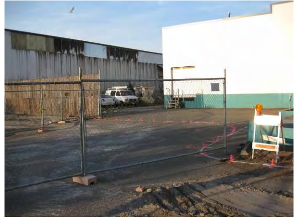
Photo 2C: Pre remediation – freeze wall alignment layout at northwest corner of Tacoma Fixtures building looking northeast.
