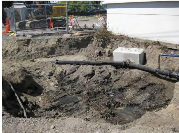
Photo 6B: Safe Dig Area excavation – looking northwest corner. Water main bypass in foreground.
