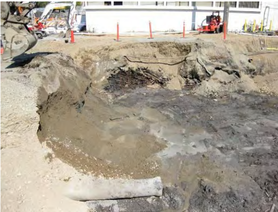
Photo 23B: Excavation area - west end looking north. Orange sewer bypass pump for Tacoma Fixtures in upper right of photo. Note: storm line protruding from west sidewall.
