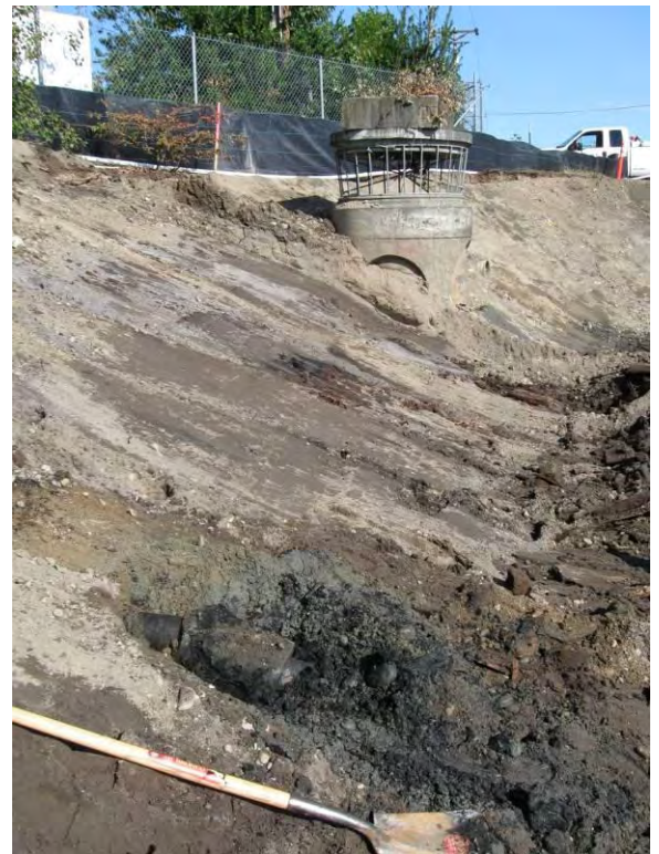
Photo 24A: 4-inch pipe in west sidewall of the north WSDOT pond looking north.
