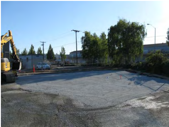
Photo 9D: Grading – gravel base for new asphalt. North end of excavation area looking southwest.
