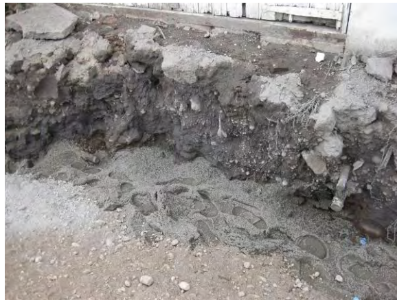
Photo 13B: Steel fuel pipes – pipes cut and plugged with cement are protruding from sidewall at the right and left center of photo.
