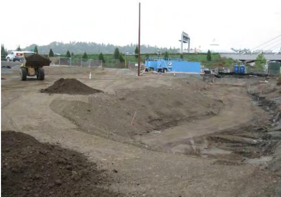
Photo 23A: Excavation backfilling – WSDOT pond subgrade reconstruction. North end of excavation area looking south.
