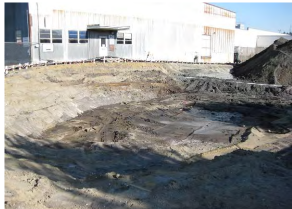
Photo 16C: Excavation – north end looking southeast toward SuperValu building, soil fill removed down to top of groundwater table.
