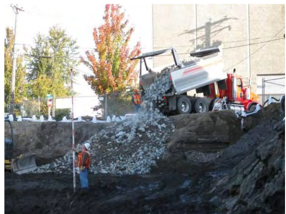
Photo 38C: Excavation backfilling – placing quarry spalls at the north end of excavation area.
