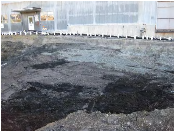
Photo 17C: Excavation – freeze wall along west side of SuperValu building. Wood waste exposed in base of excavation.
