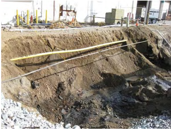
Photo 32B: East 19 th Street UST – UST removed with bank run backfill in north sidewall from Safe Dig Area. Note: natural gas main and telecom line crossing tank pit supported with temporary guy lines.
