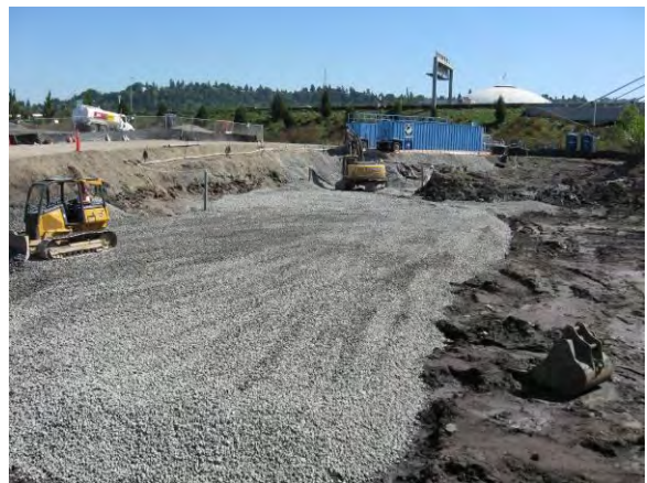
Photo 20A: Excavation backfilling – placing ballast across excavation base. North end of excavation area looking south.
