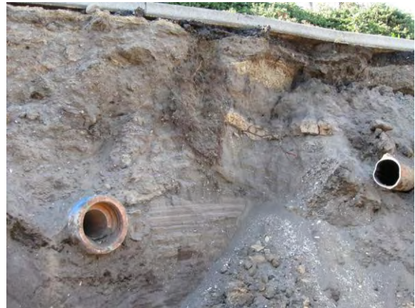
Photo 4D: BNSF Oil Pipeline to the right and storm sewer line to the left looking northwest.
