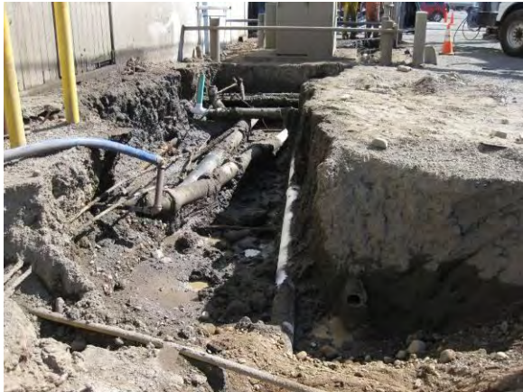
Photo 10B: Safe Dig Area – underground utilities exposed along north side of excavation looking east.
