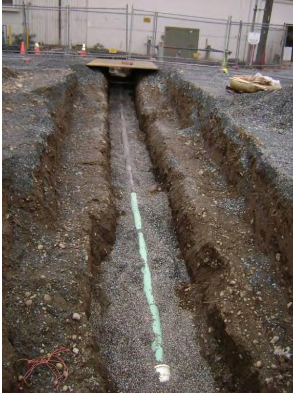
Photo 50B: Utility reconstruction – Tacoma Fixtures sanitary sewer lateral crossing East 19 th Street.
