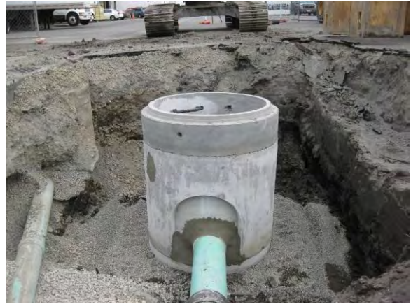
Photo 45B: Utility reconstruction – new sanitary sewer manhole at southeast corner of Area B with bypass system looking east.
