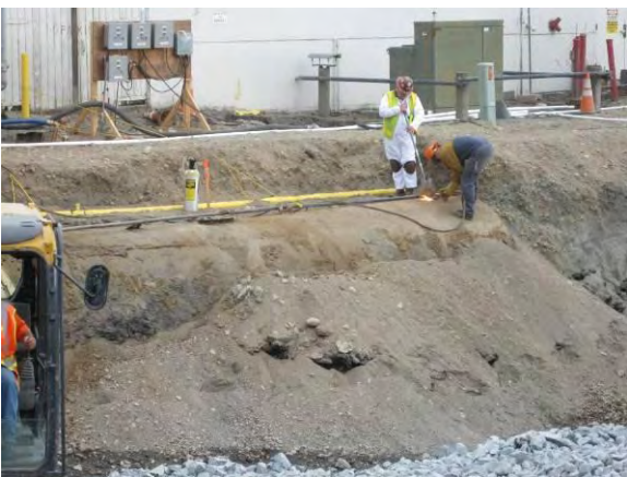
Photo 25B: East 19 th Street UST - cutting UST with torch while marine chemist monitors tank atmosphere.
