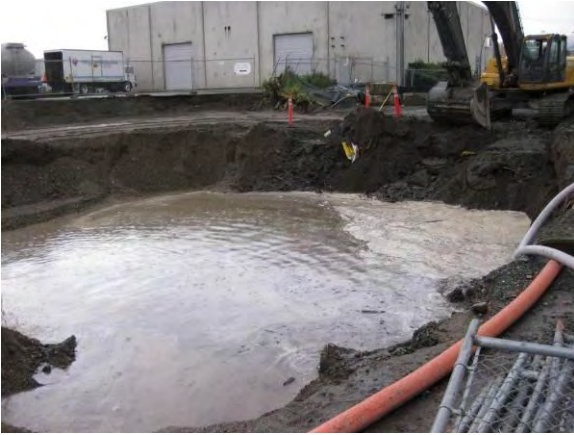
Photo 44B: Northwest corner of excavation area west of Phoenix lay down yard, looking southeast. Note: base of excavation is 6 feet below water surface.
