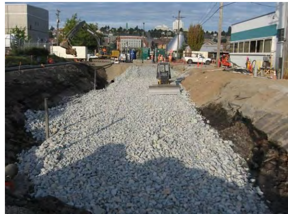
Photo 58B: Excavation backfilling – placing quarry spalls across base of excavation looking west.
