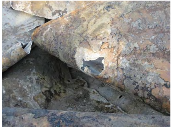
Photo 33B: East 19 th Street UST – Note: observed fist-sized holes corroded through side of UST.
