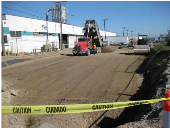
Photo 62B: Excavation backfilling – placing next lift of bank run backfill, southwest corner of excavation looking northeast.
