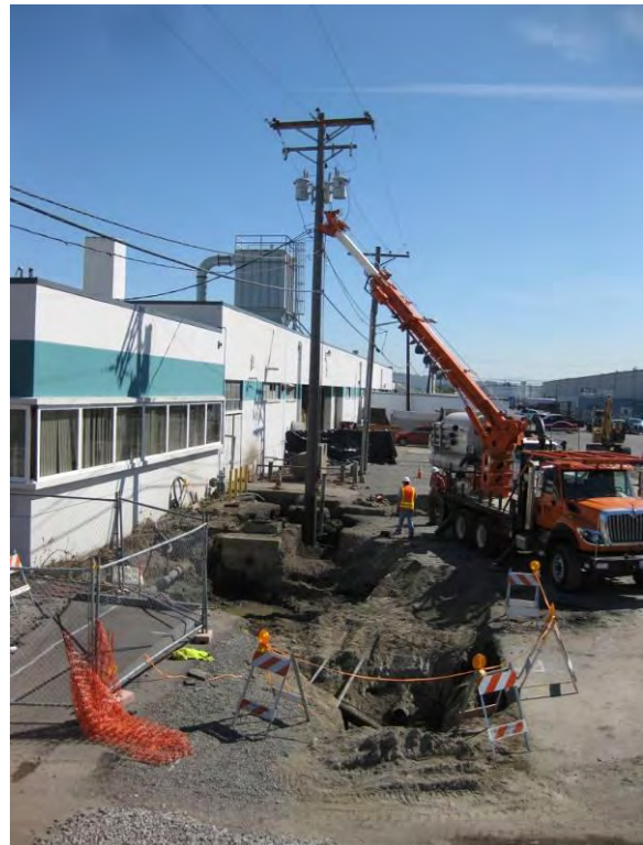
Photo 8B: Safe Dig Area – Tacoma Power boom truck holding power pole during excavation activities.
