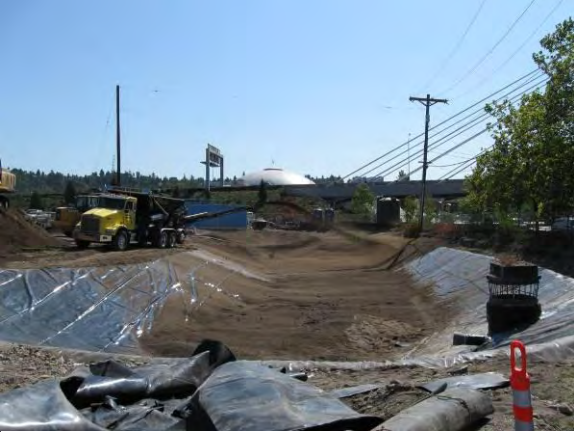
Photo 25A: Pond rebuilding – placing pond surcharge material over pond liner. North end of excavation area looking south.
