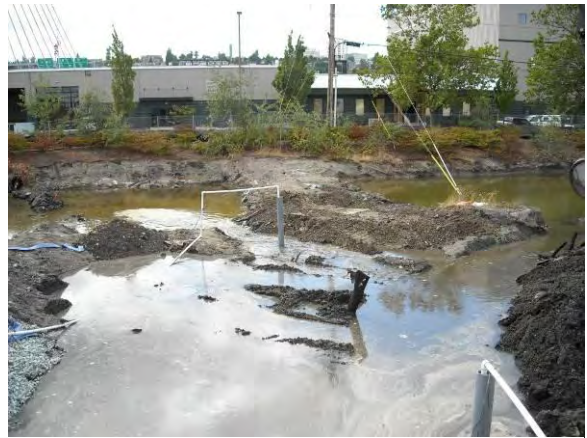
Photo 10A: Excavation dewatering – south half of excavation area looking west. Gray PVC dewatering sumps center and bottom right of picture.
