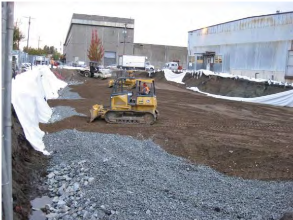
Photo 41C: Excavation backfilling- north half at north end of excavation area looking north.
