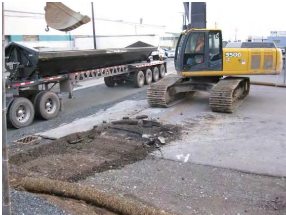
Photo 38B: Nichols area excavation – beginning in southeast of Area B looking northeast.
