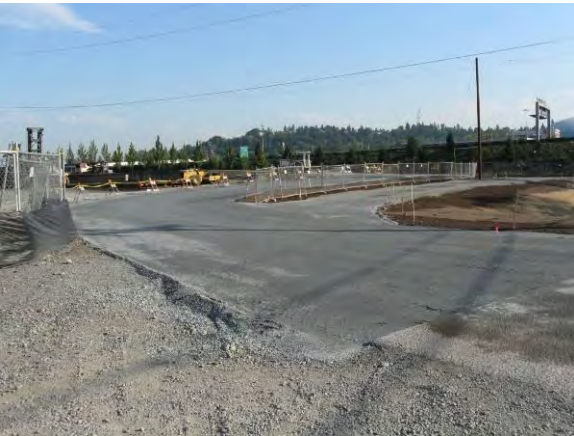
Photo 27A: Site grading – subgrade placed for asphalt access road. Northwest corner of excavation area looking southeast.
