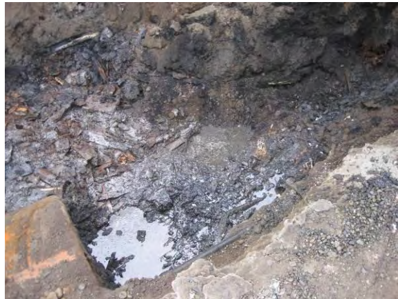
Photo 11B: East 19 th Street UST – east end of UST within Safe Dig Area.
