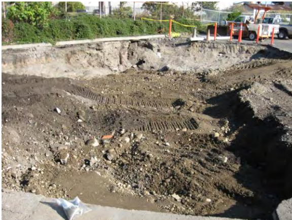
Photo 7D: Backfilling – bank run fill placed in lifts south of excavation area end looking north.
