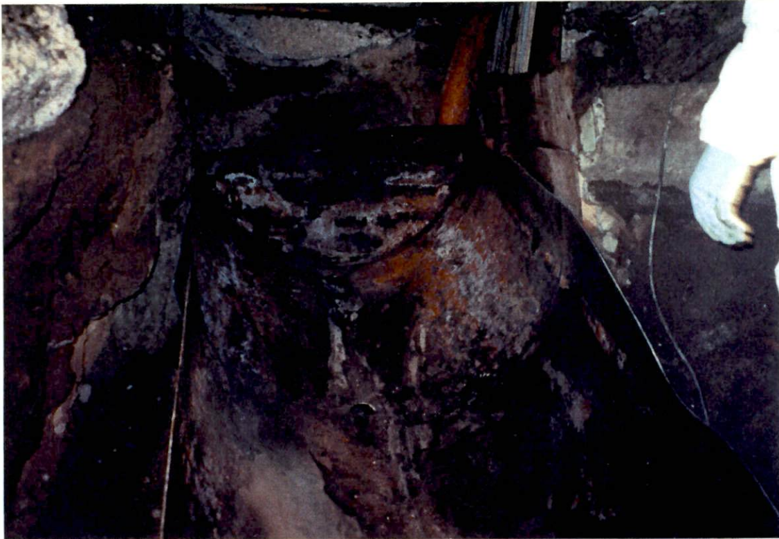
Photograph 13 (above) – Lower half of UST1.
