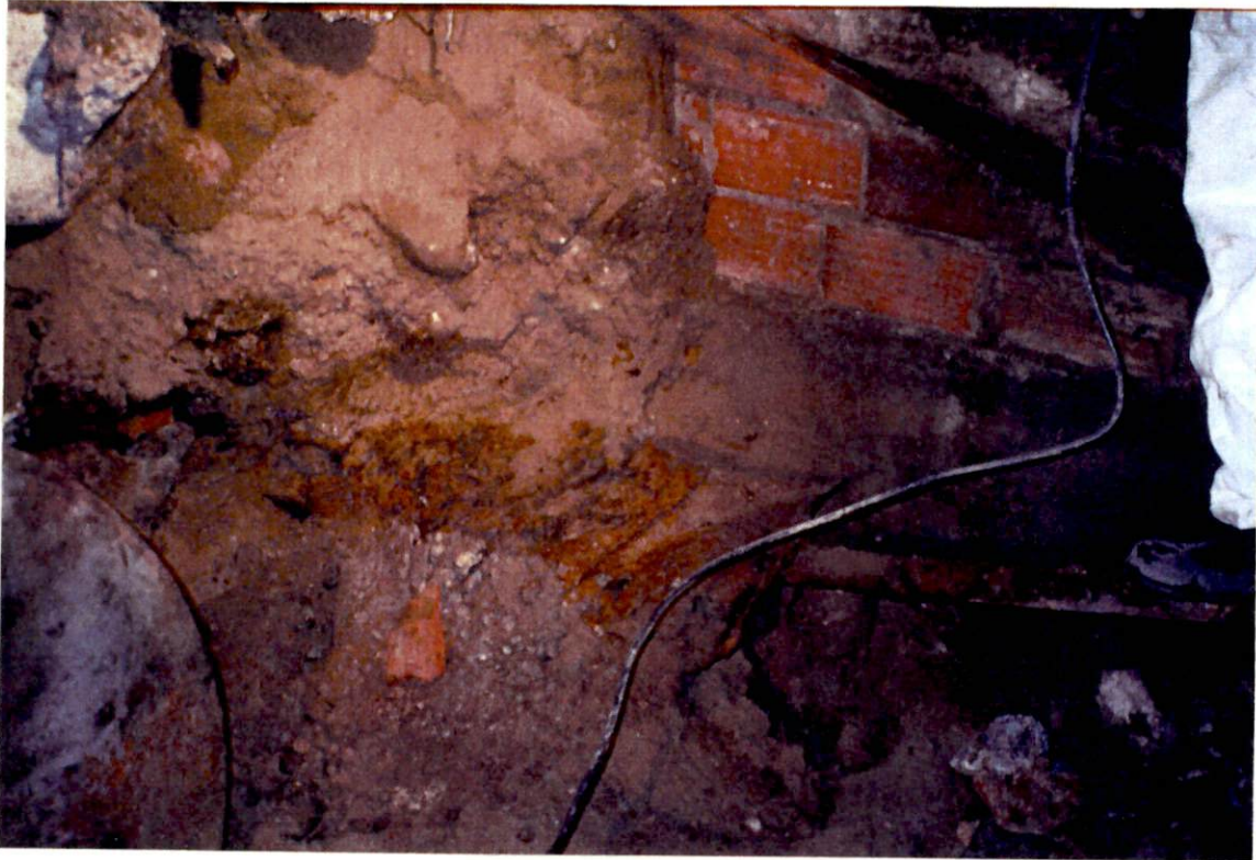
Photograph 7 – Miscellaneous debris in upper 2-feet around UST1.
