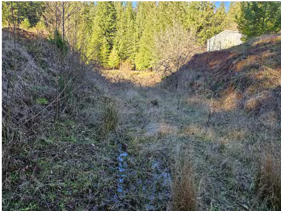
Photo 26. Drainage from the western sewage lagoon breach.
