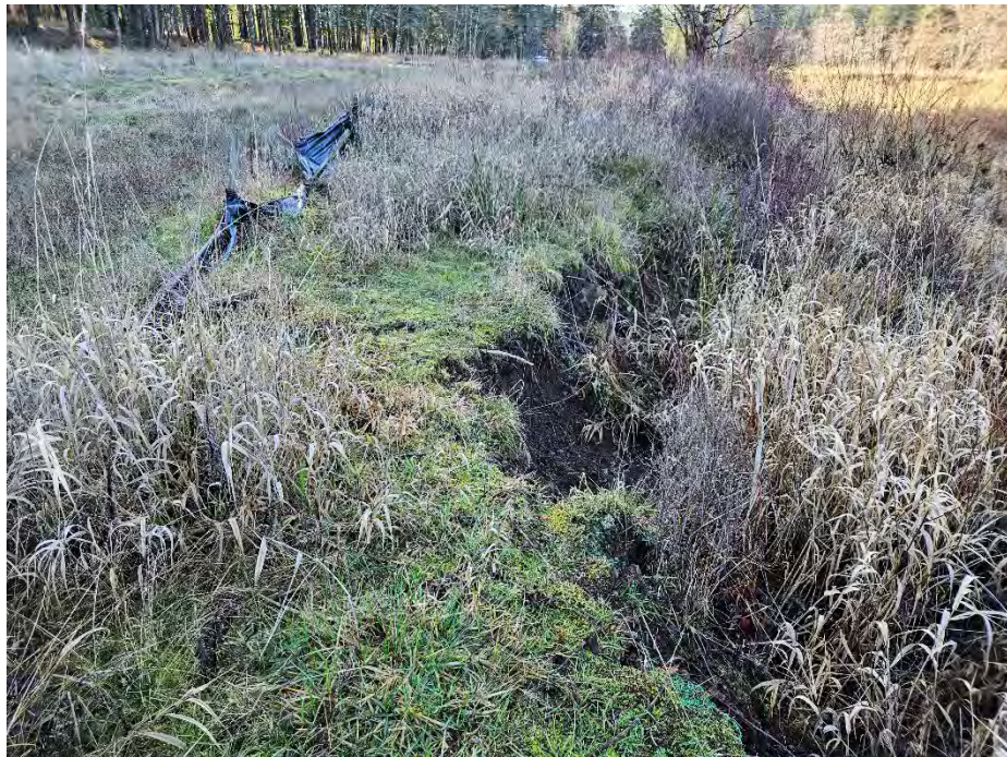
Photo 18. RAU-2A-16 soil cap area: bank erosion 4.5 feet from soil cap.
