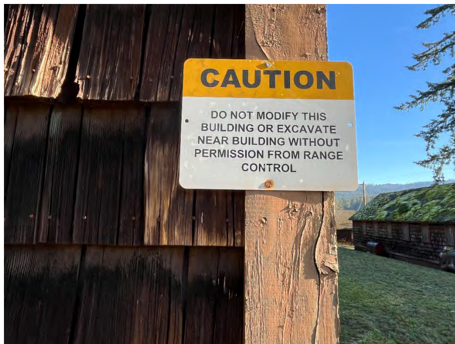
Photo 15. Building T-1932 AST signage.
