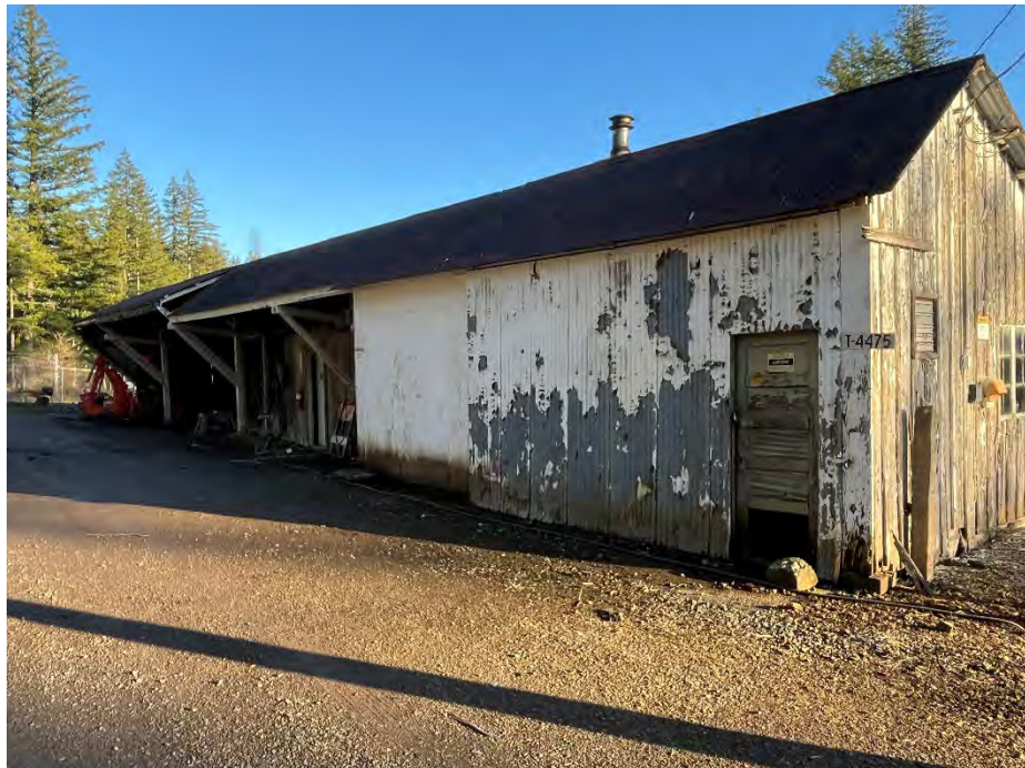
Photo 10. Building 4475 maintenance pit area signage.
