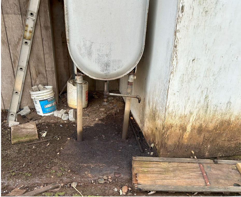
31. Presumed oil staining at exterior of Bldg. 4475
