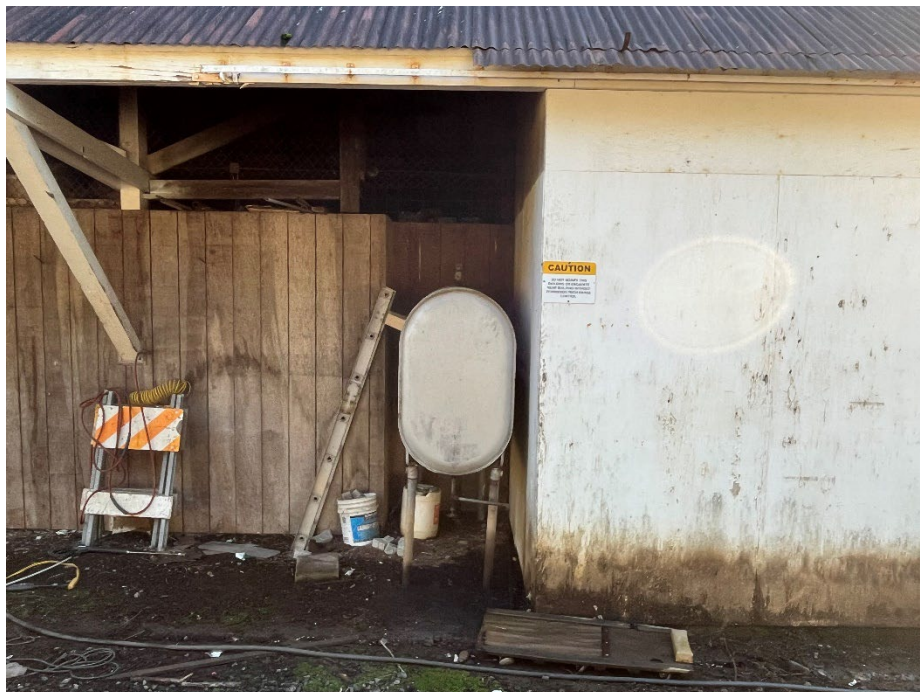
Photo 12. Building 4475 maintenance pit area signage
