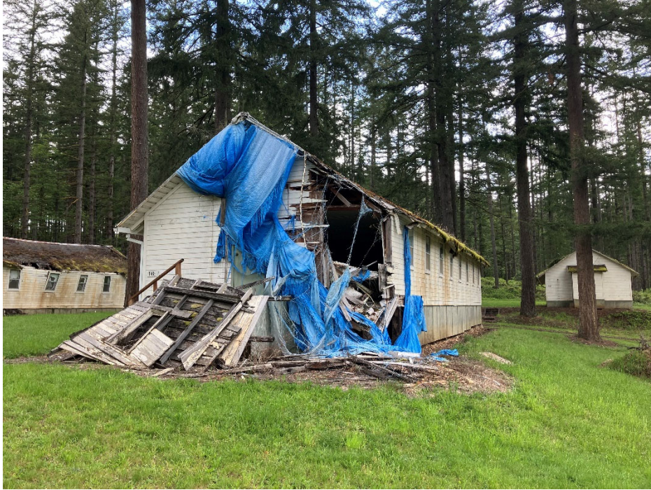
26. Camp Killpack cantonment – Damaged building. County is planning to demolish unsafe structure.
