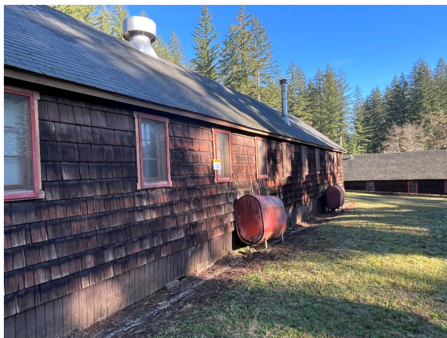
Photo 14. Building T-1932 AST signage
