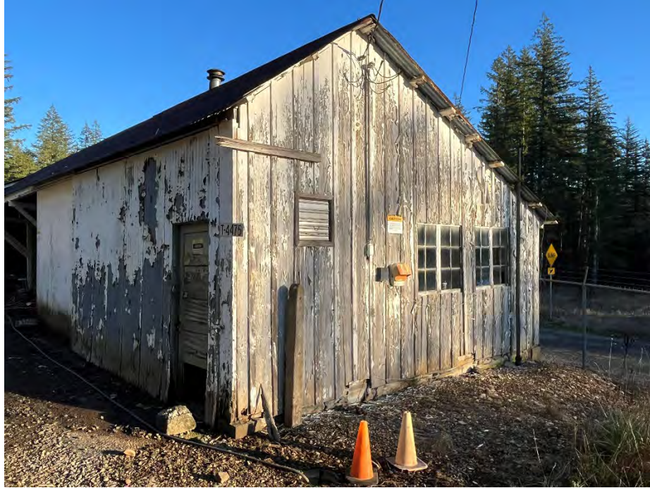
Photo 11. Building 4475 maintenance pit area signage.
