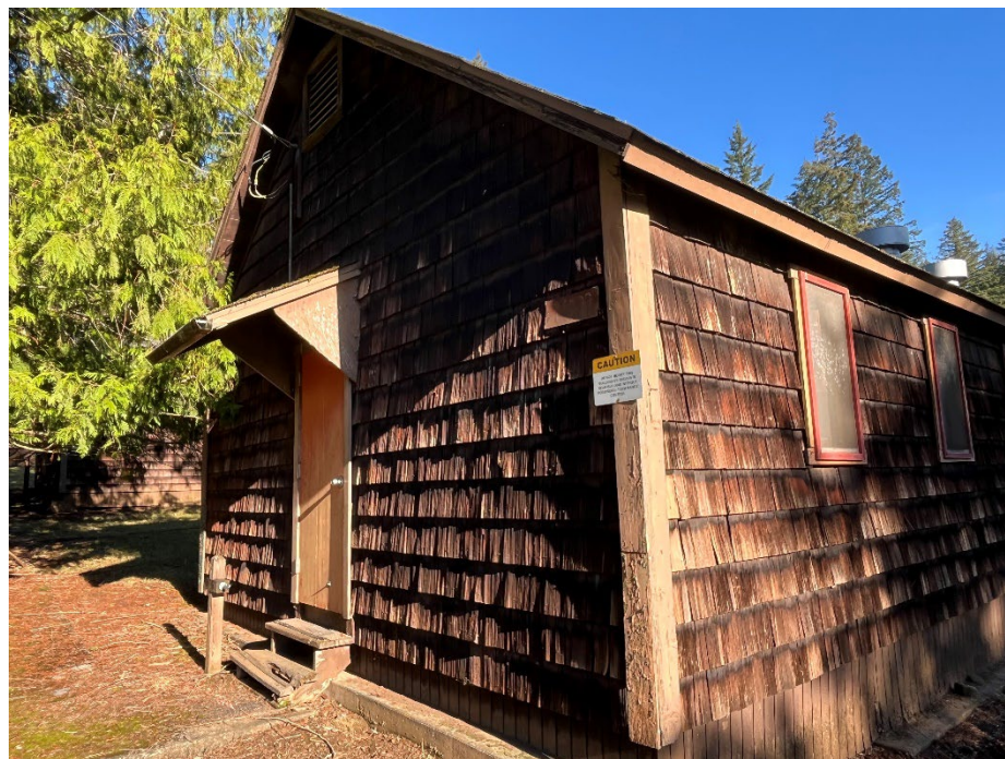
Photo 13. Building T-1932 AST signage
