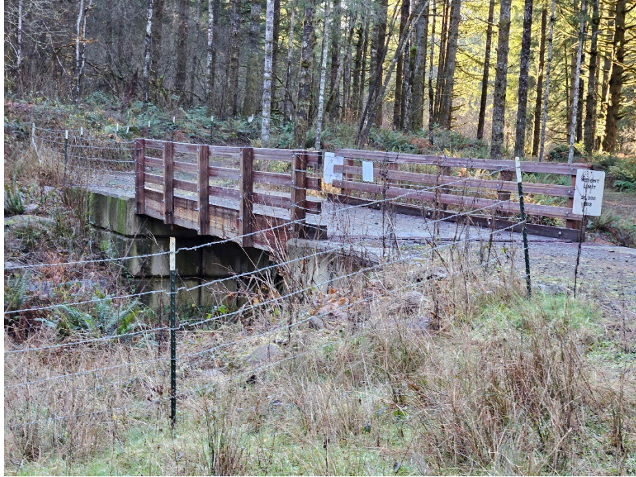
Photo 3. Five strand barbed wire at CITA expansion
