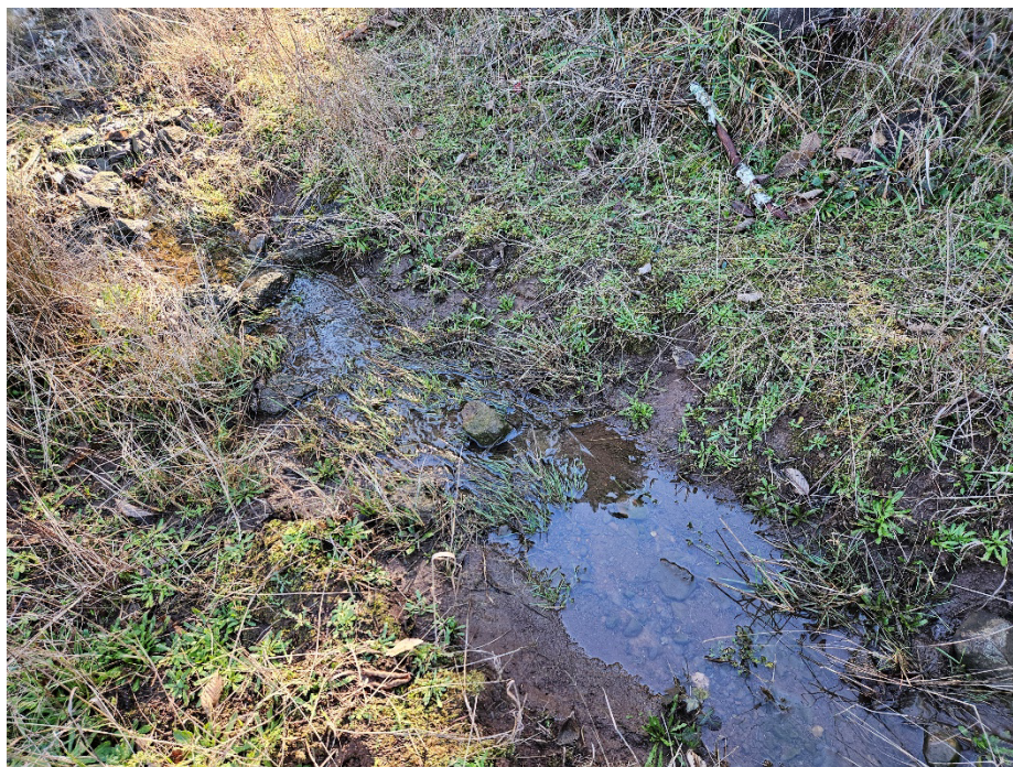
Photo 27. Drainage from lagoon breach
