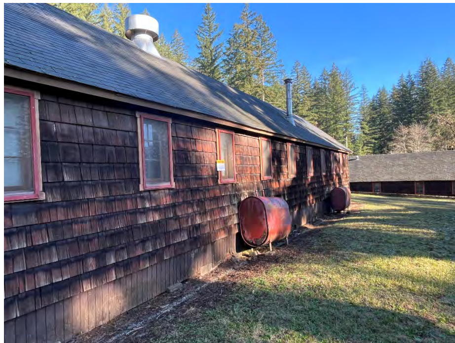
Photo 14. Building T-1932 AST signage.
