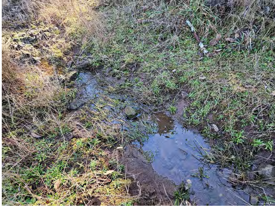
Photo 27. Drainage from the lagoon breach.
