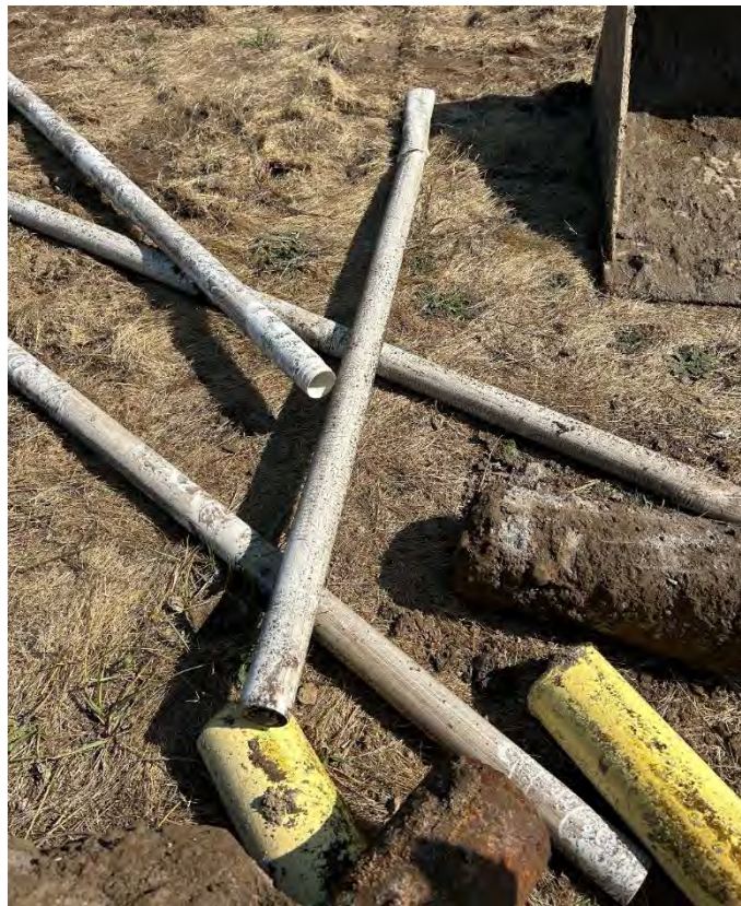
Photo 8: Image of the removed well screen from LB-6S.
