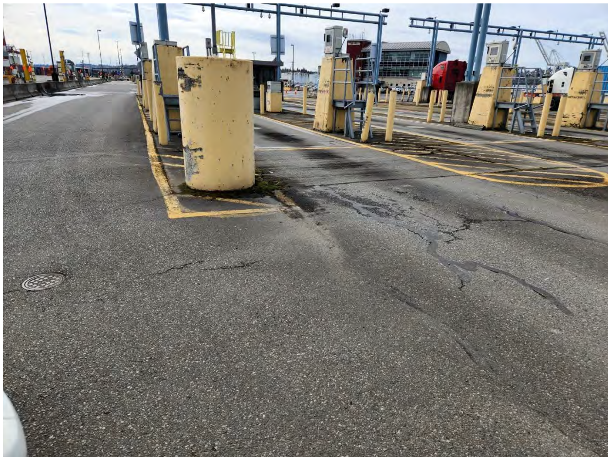
Photo 6. Terminal 18 Northern Area Pavement Cracks with Repairs
