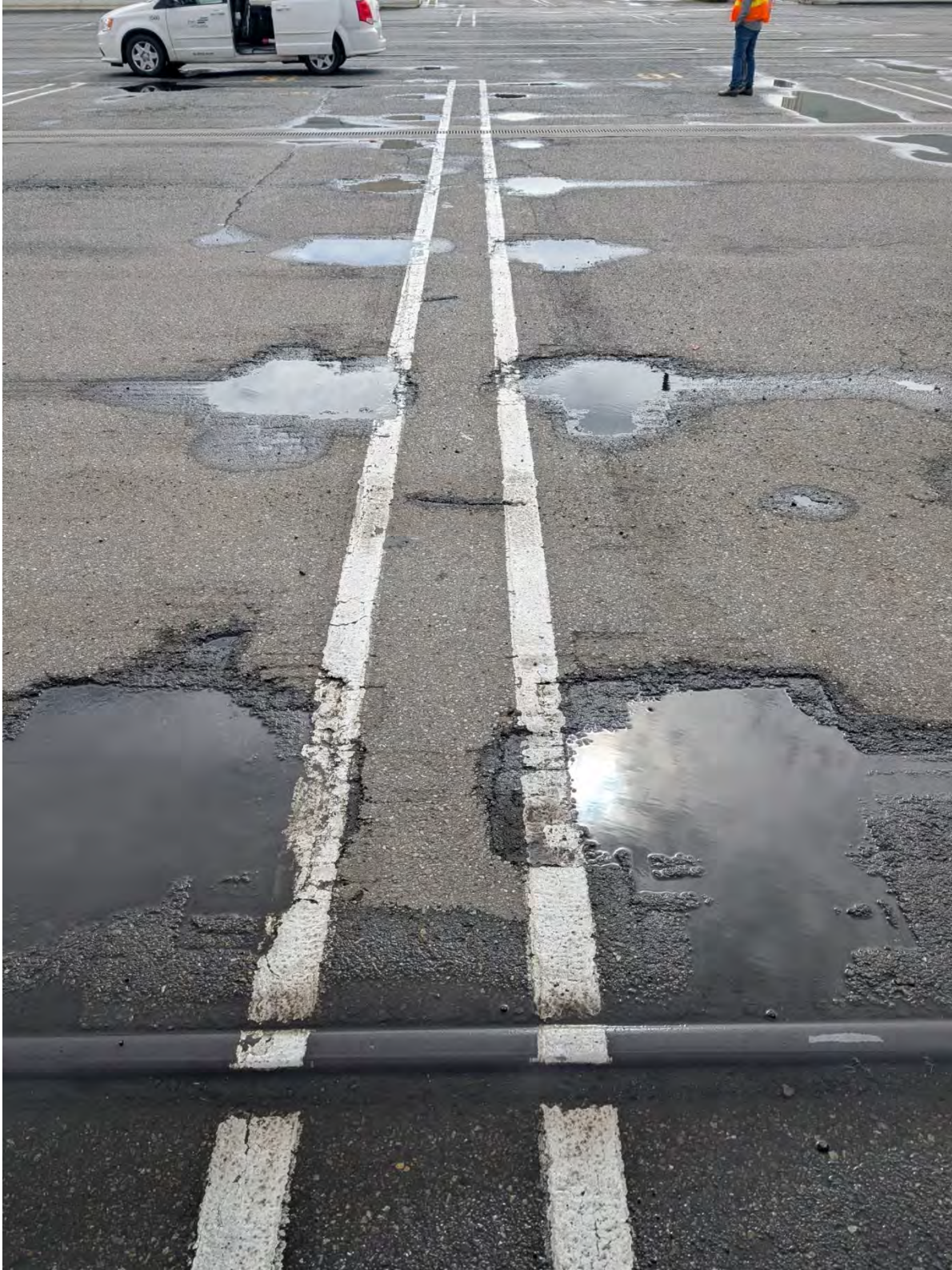
Photo 8. Terminal 18 Central Area Cap Damage from Containers
