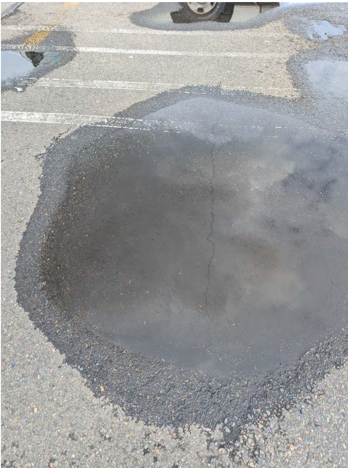
Photo 7. Terminal 18 Central Area Ponding with Cracking
