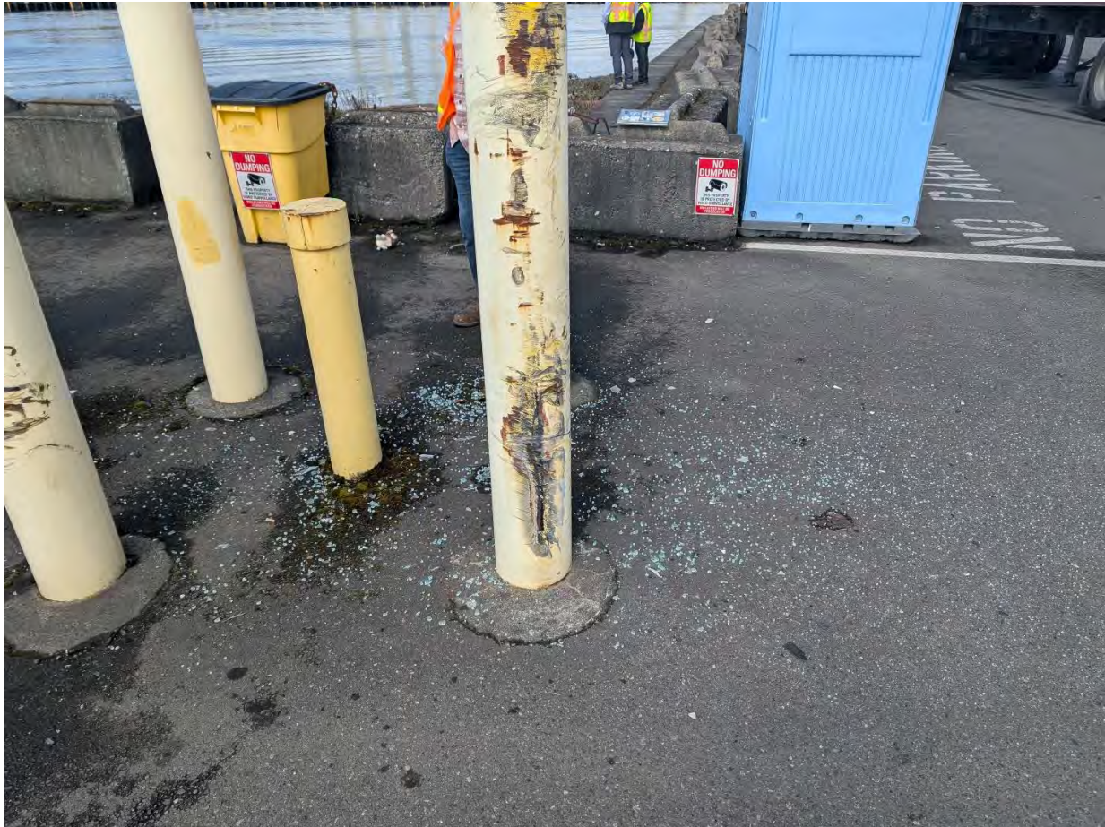
Photo 2. Lockheed Upland Monitoring Well LMW-32D with Damaged Bollard
