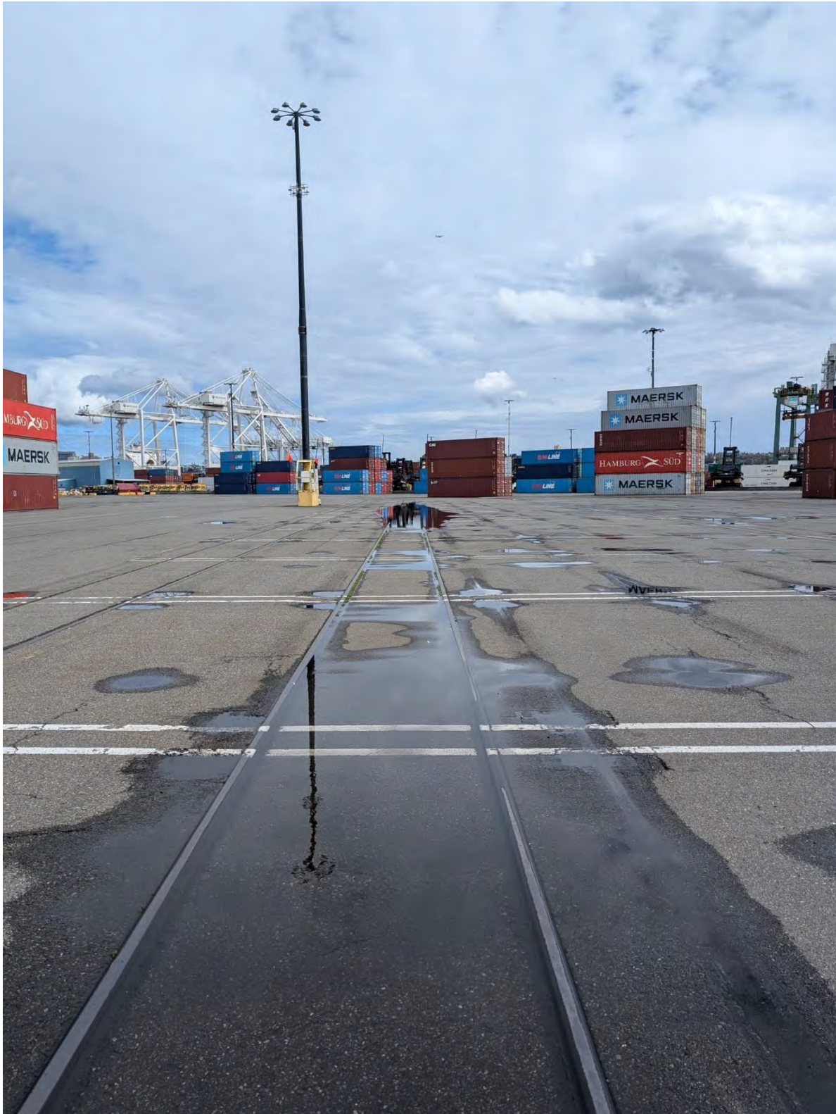
Photo 9. Terminal 18 Southern Area Ponding Along Rail Lines
