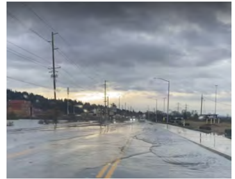
The record tide in the Tacoma Harbor caused flooding on freight corridors including local roadways and rail. The high tides kept stormwater systems from draining, causing upland urban flooding issues.
