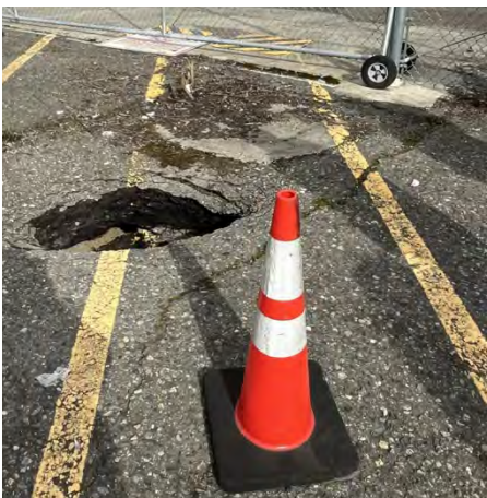
Terminal 46 sinkhole (shown above)
