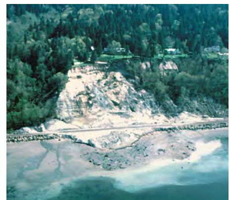
The 1997 Woodway landslide affected the railroad corridor between Seattle and Everett, derailing freight cars on a passing train and temporarily halting rail operations.
