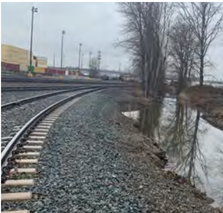
Bullfrog Junction Ditch (shown above) in the Tacoma Tideflats is a critical link between rail in the Tideflats and the mainlines. Urban flooding issues here have caused flooding on nearby properties and have the potential to disrupt rail operations.
