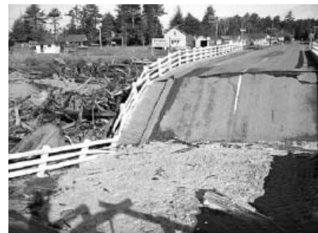
Distant source tsunami waves from the Great Alaskan Earthquake destroyed a bridge on the Washington outer coast.
