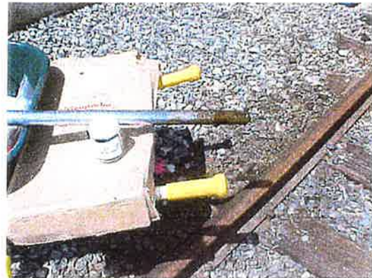
Boring B15 location. Note (free) oil coating on end of push probe after being pushed to one-foot depth.
