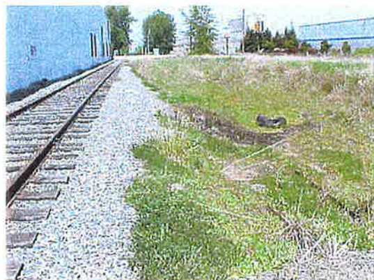
Ground staining and distressed vegetation were present near the B15 location where shallow free product was present. View looking north.
