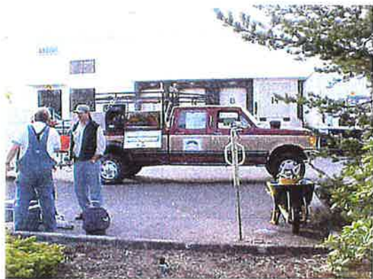
Drilling with the push probe at Boring B10, the inferred up-gradient boring. Note the patching of the asphalt blacktop near the standing personnel.
