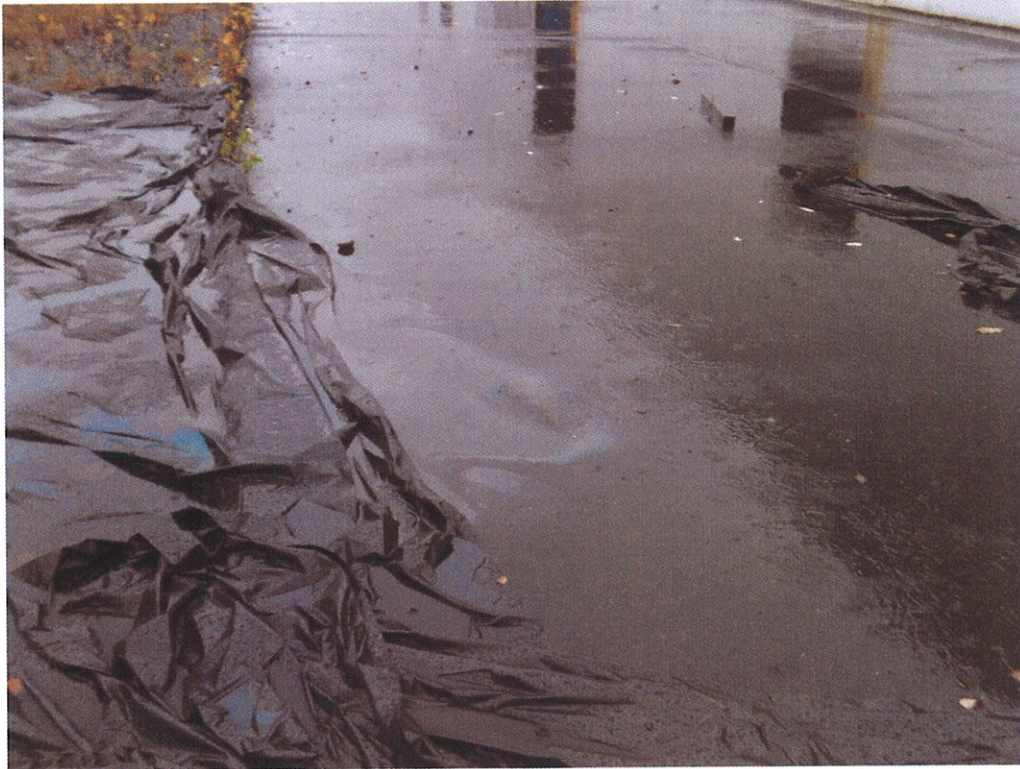
View looking south, note the slight sheen accumulation near the pavement edge downgradient of the hydraulic oil release area. This sheen is from typical parking lot runoff from an upgradient area.
