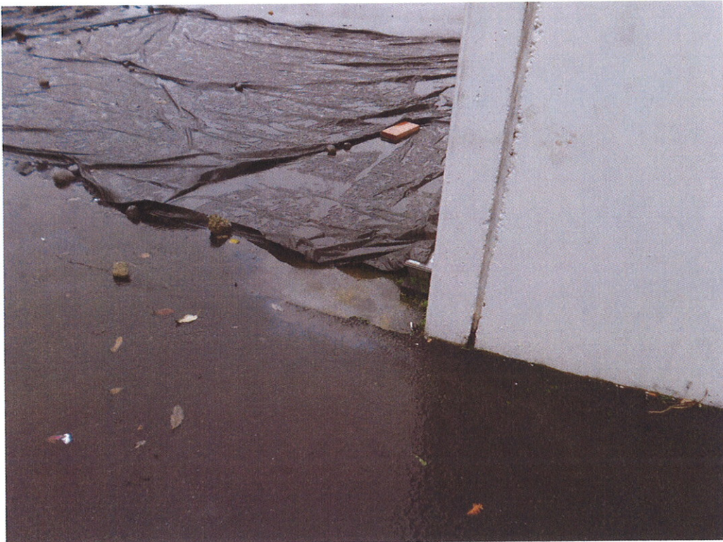
View of the northeast corner of the Manufacturing Building. Note the slight sheen from typical parking lot runoff flowing towards the hydraulic oil release area from the upgradient asphalt paved area.
