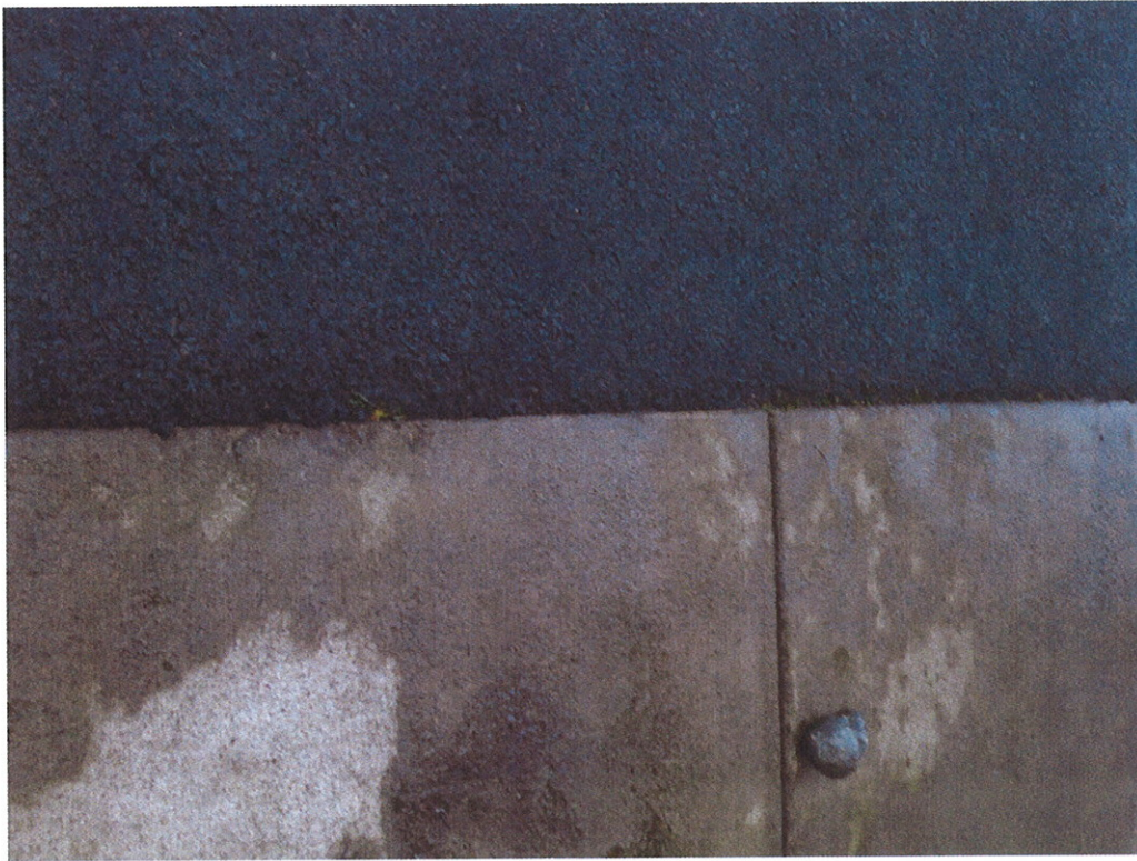
View of the joint between the concrete walk and the asphalt pavement below the overhead door in the Baler area. Joint integrity is good. Note lack of staining. Soil boring SB206 collected at this location.
