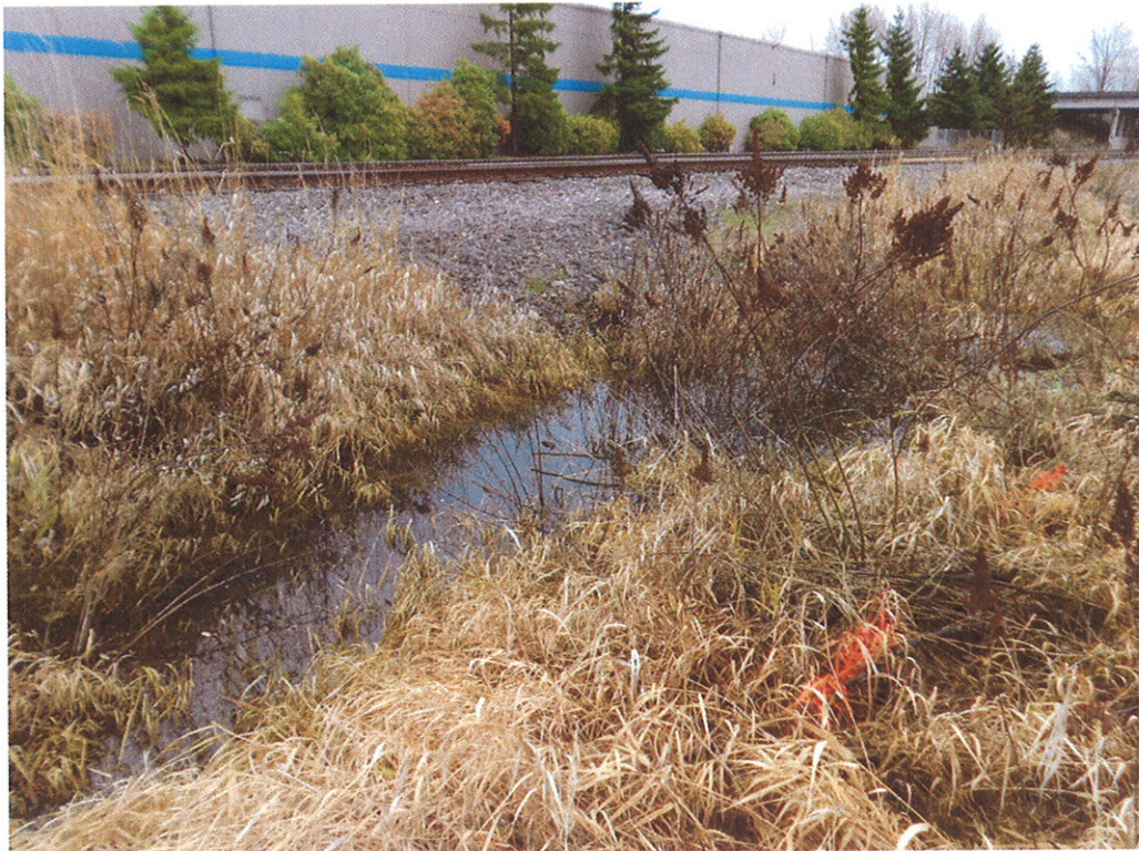
View looking southeast from the excavation area at the drainage swale approximately 20-feet (centered) east of the excavation edge. No sheen observed.
