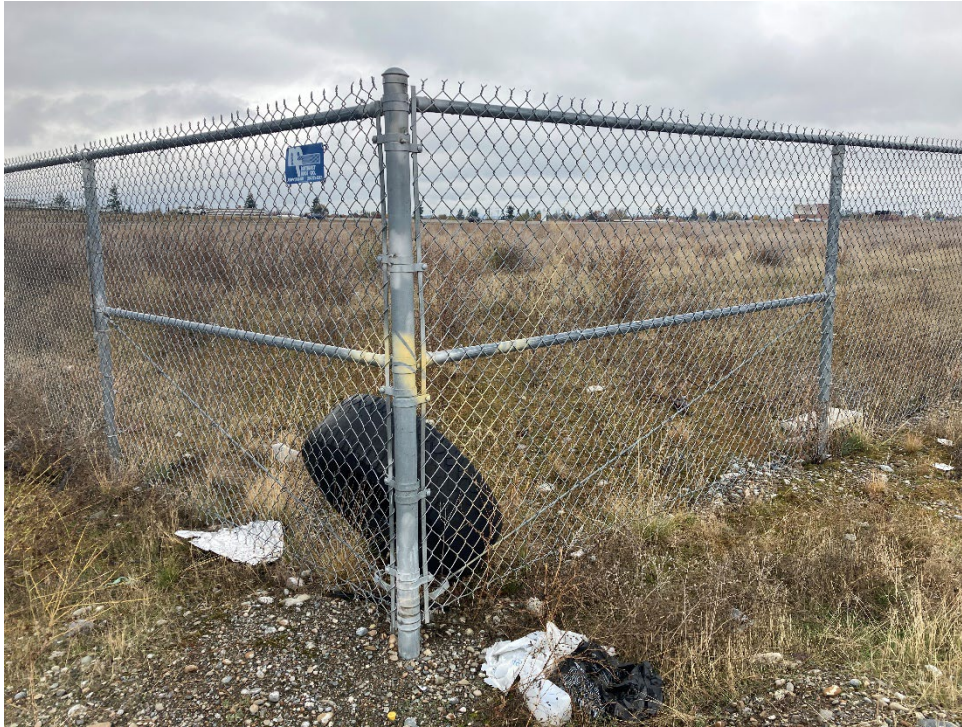
Photo 5: Southeast corner of perimeter fence with debris — from the southeast
