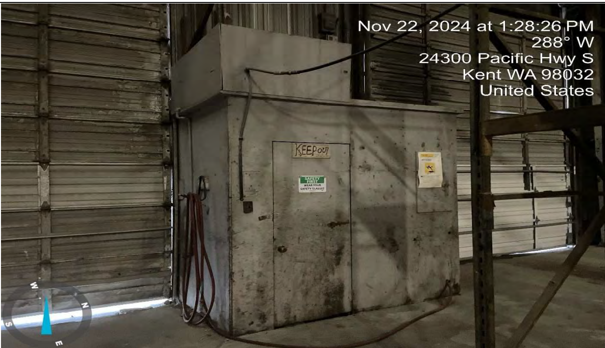
24. Air compressor room on western side of maintenance garage building (Viewing W-NW)
