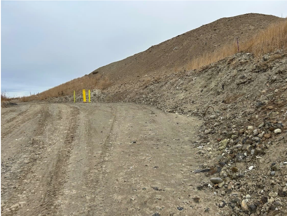
Thermistor T-4 Installation Access
