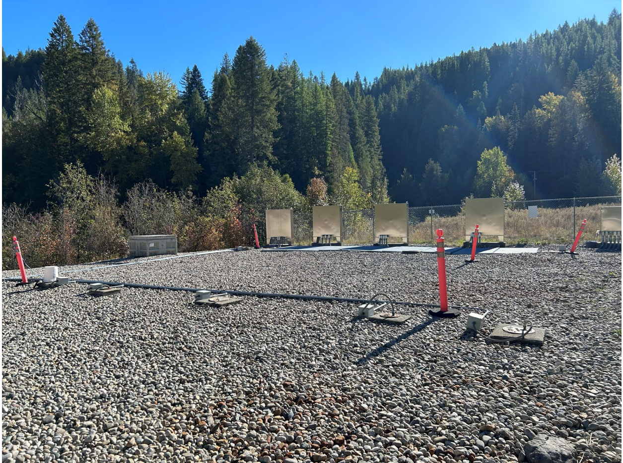
Photo 1: Groundwater remediation system – gate treatment area
