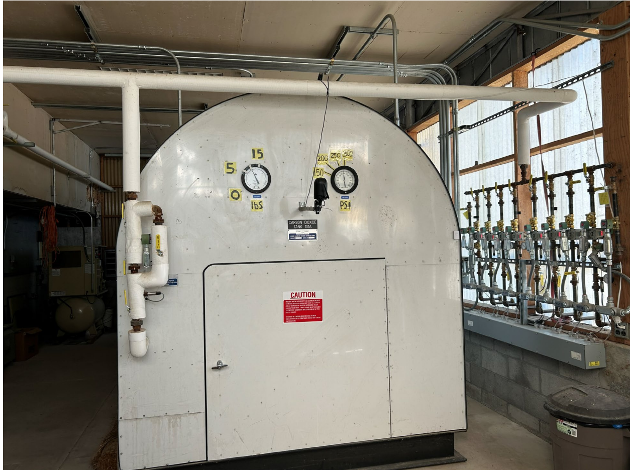
Photo 2: Tank and piping within the support building
