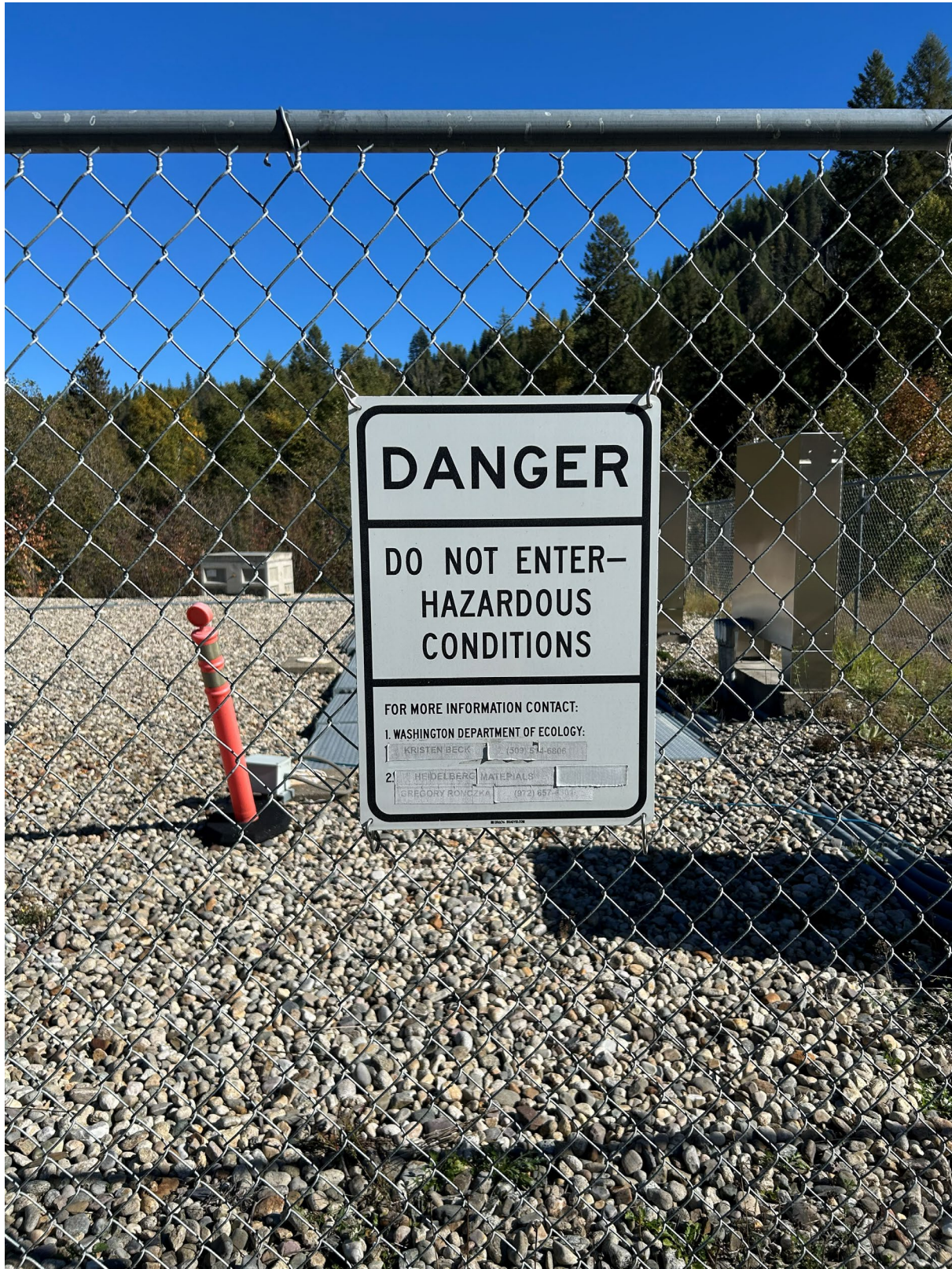
Photo 4: Signage on groundwater remediation system
