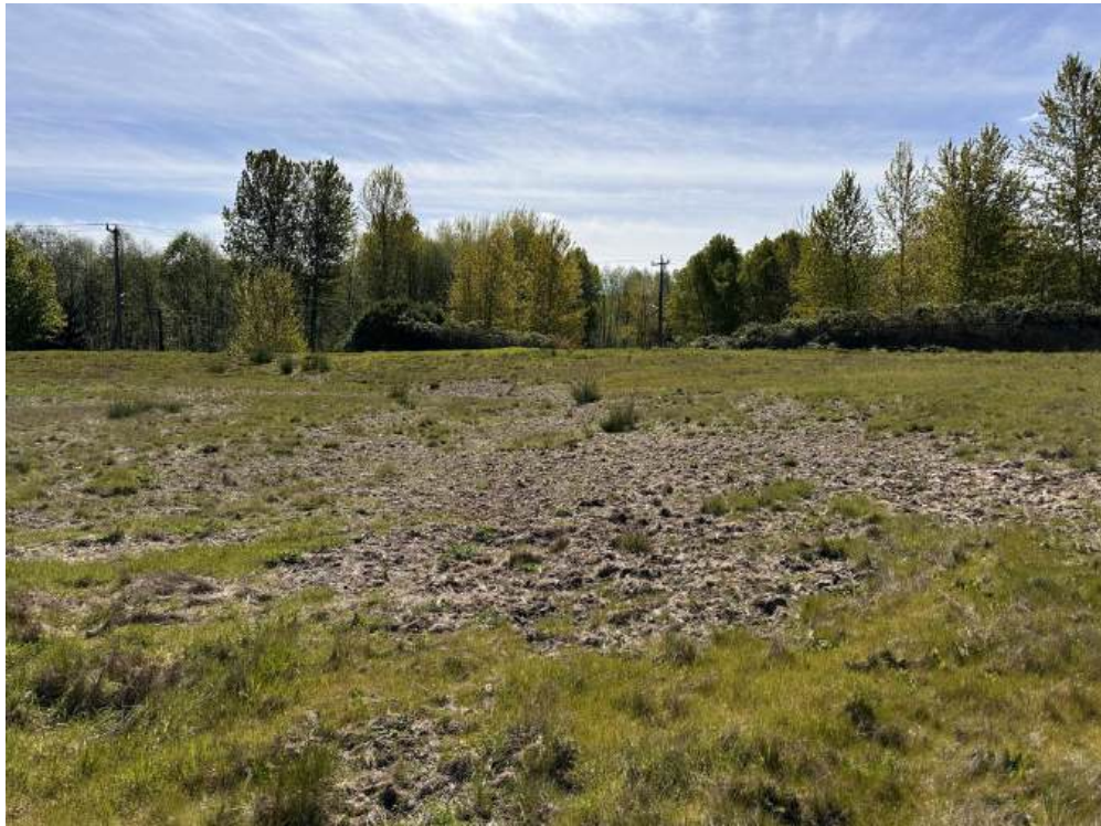
Photograph L18. Station LLA 18. Exposed underlying soil and loss of barrier material.
