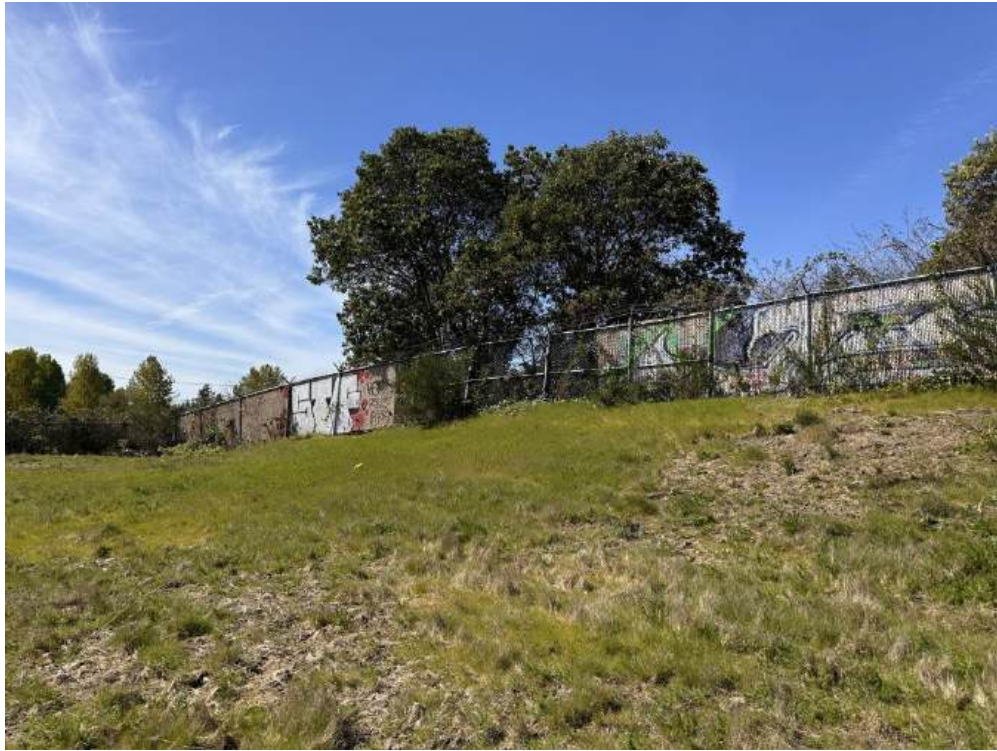
Photograph L13. Station LLA 13. Exposed underlying soil and down-slope movement of barrier material.
