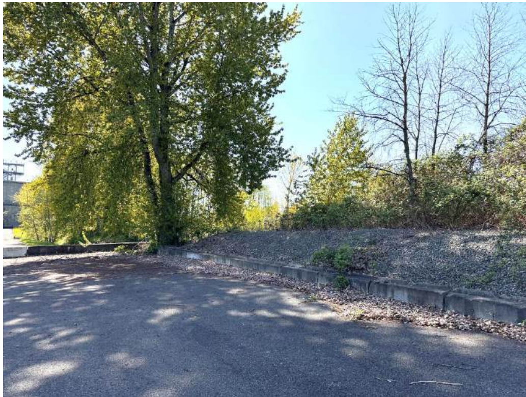
Photograph D9. Station DMCA 09. Presence of debris on barrier surface.
