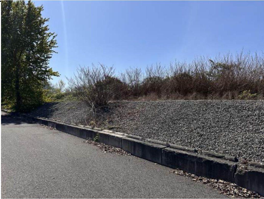
Photograph D1. Station DMCA 01 in good condition with some debris on barrier surface.
