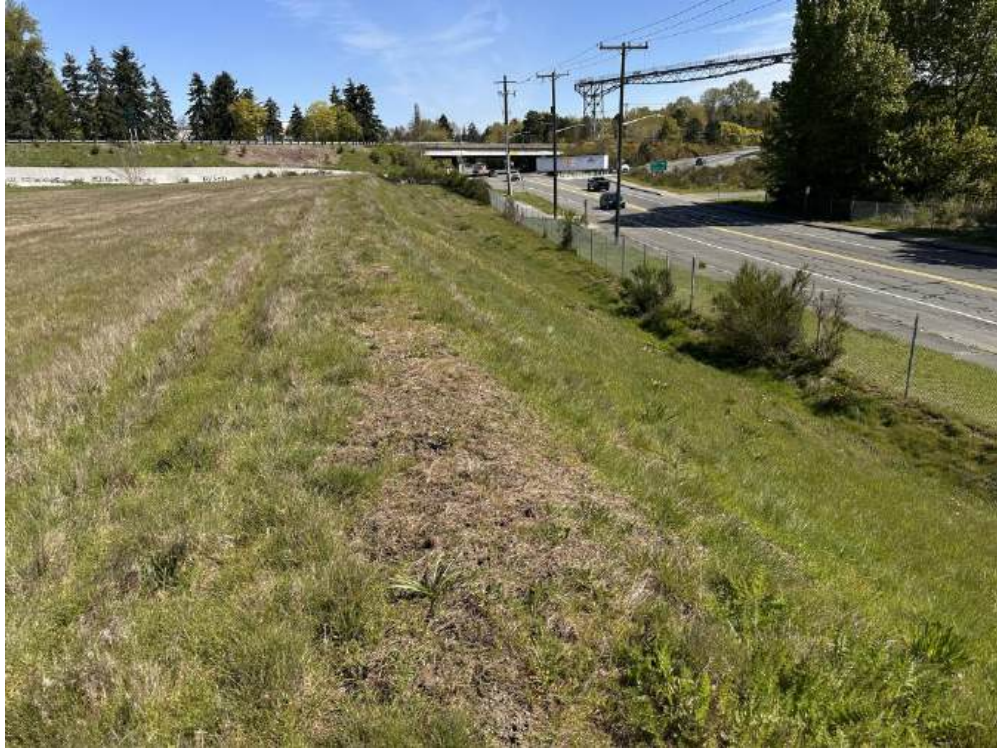
Photograph L17. Station LLA 17. Exposed underlying soil and down-slope movement of barrier material.
