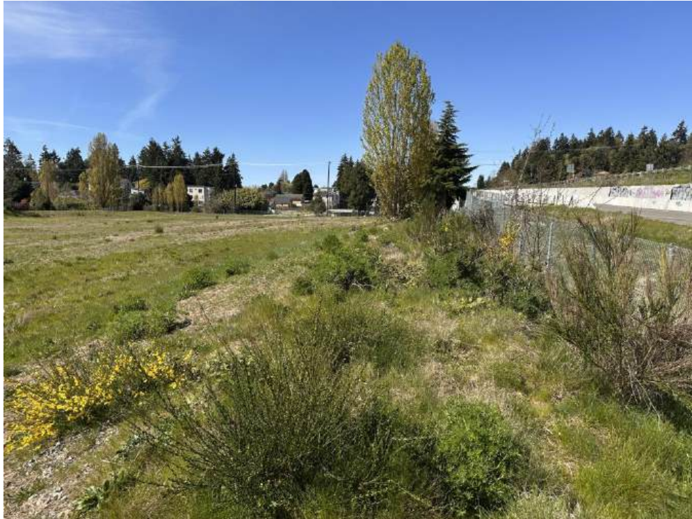
Photograph L5. Station LLA 05. Loss of barrier material and substantial plant growth.
