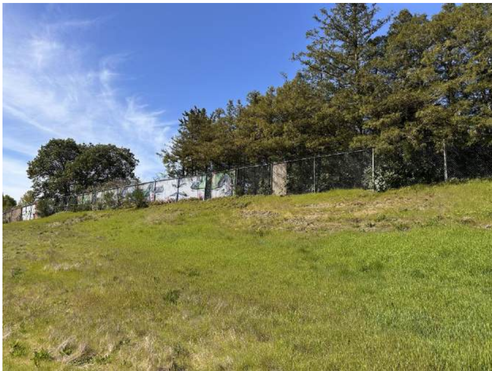
Photograph L12. Station LLA 12. Exposed underlying soil and down-slope movement of barrier material.
