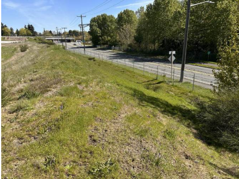
Photograph L15. Station LLA 15. Exposed underlying soil and down-slope movement of barrier material.
