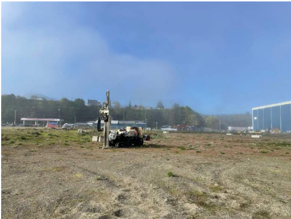
Figure 9. View of boring G8, looking south. Note boring within 2015 mass excavation area.
