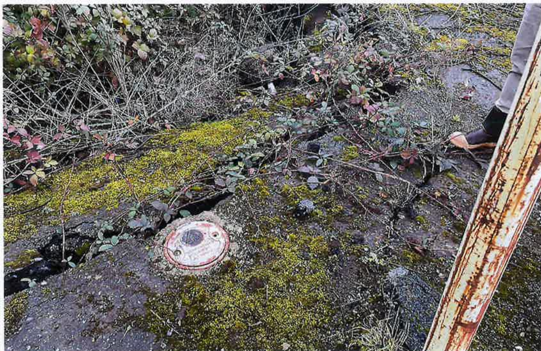
Photo 6: Well MW-1203R looking northwest, toward the Snohomish River. Slope failure can be seen adjacent to the well.
