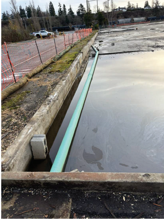
Photo 19: Ponding post pumped North truck bay to CB (see Photo 20)
