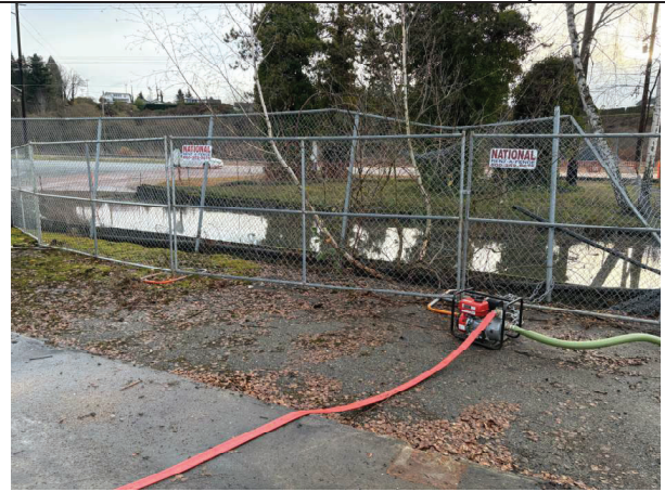
Photo 2: North Truck Bay pumping setup
