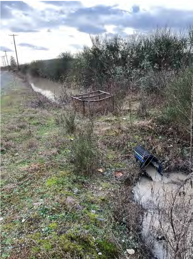
Photo point 1 Looking south at stormwater outfall and ditch from the south.
