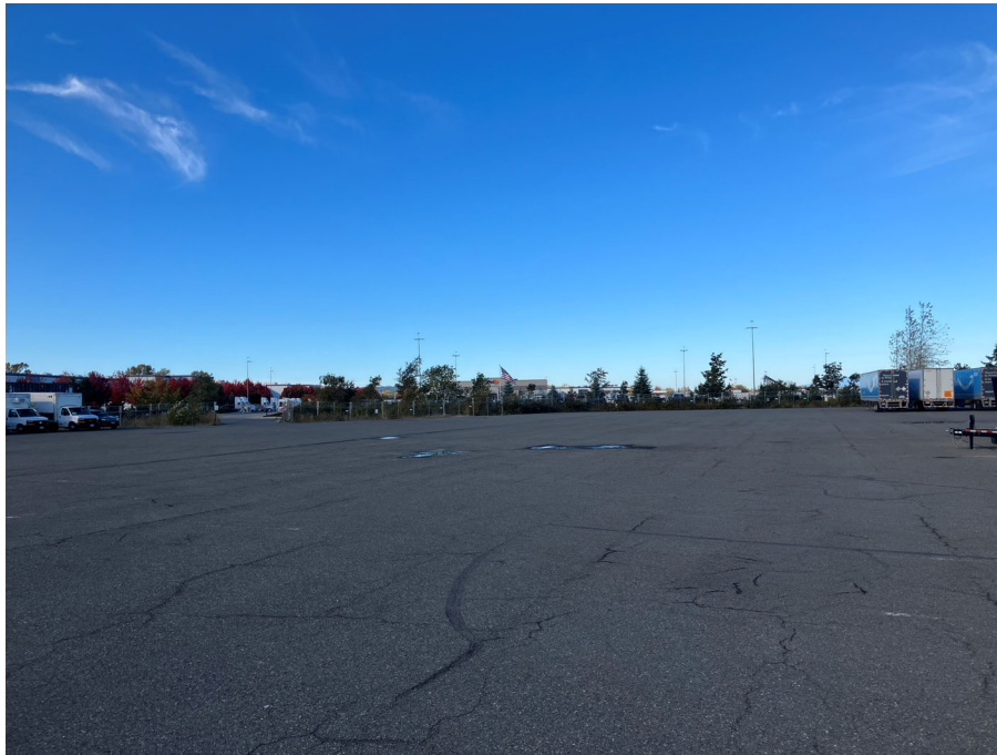
Photograph 3 - Looking northeast at central portion of the asphalt cap. Photograph shows repaired cracks and minoring ponding on asphalt cap surface. Photograph of typical asphalt crack repaired with a joint sealant.
