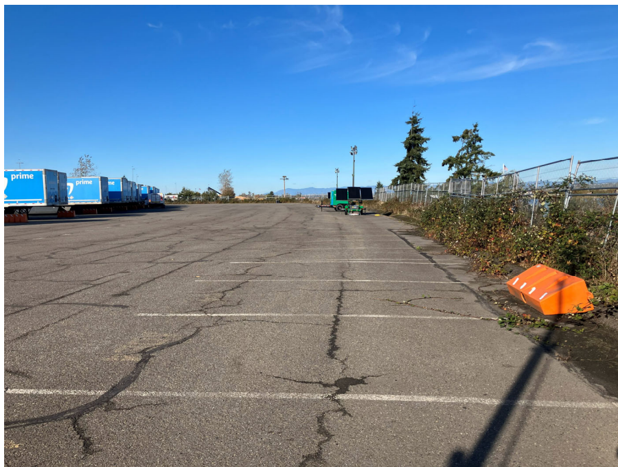
Photograph 6 - Looking north at the eastern portion of the asphalt cap. Photograph shows parked dry van trailers, and cracks, majority repaired, and vegetation growing over the asphalt cap surface.
