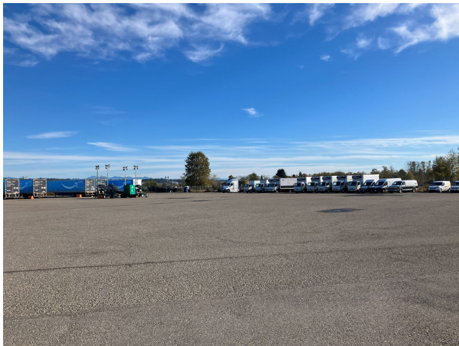
Photograph 2 – Looking southeast at southern and central portions of the asphalt cap. Photograph shows repaired cracks and minor ponding on asphalt cap surface.
