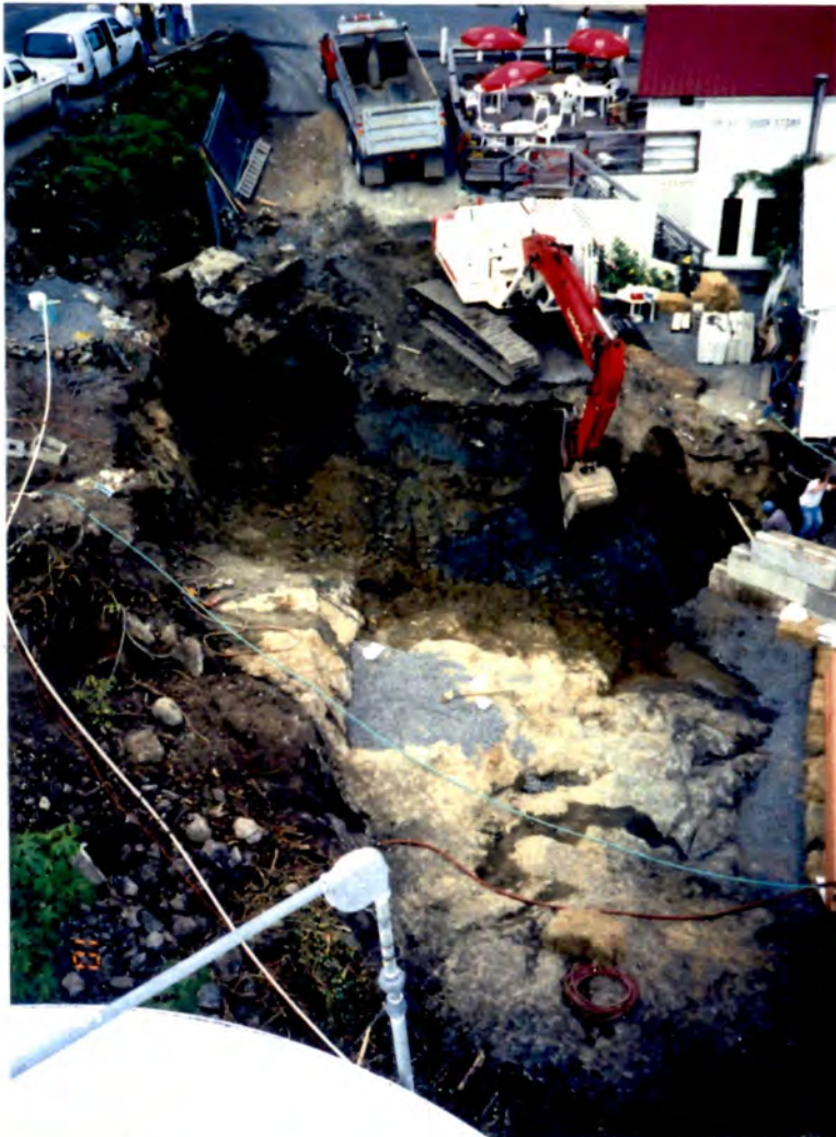
1. View looking east showing exposed bedrock contact with soil and cross section look at contaminated soil ← (gray soil).
