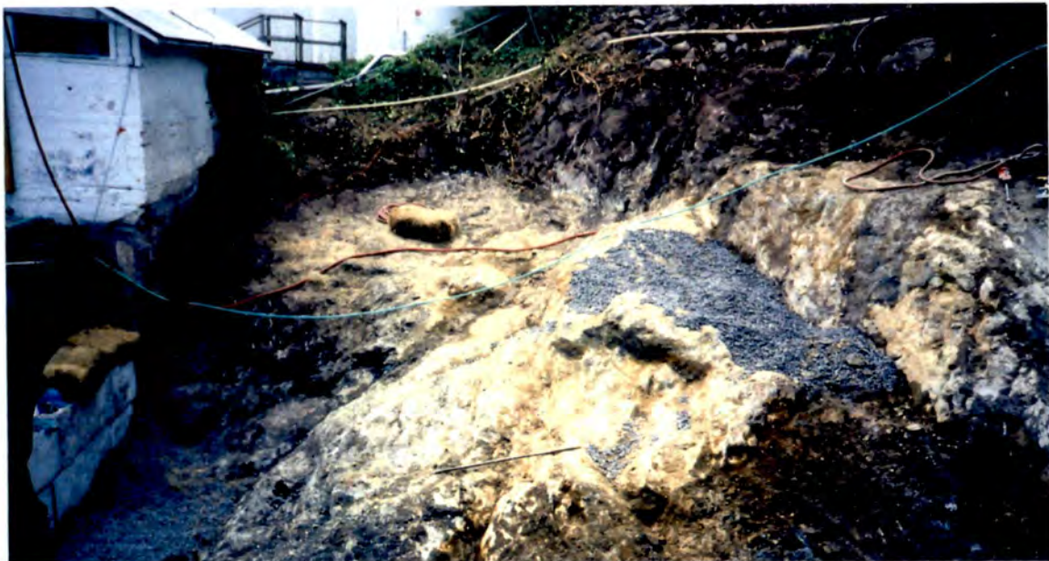
2. View looking west showing exposed bedrock storage building and removed portions of dock on left side of photo. ↓
