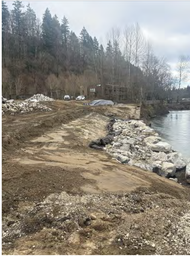
Pic 3. Clay placed over section of high-pH soil within 2 feet of the final slope, looking east.
