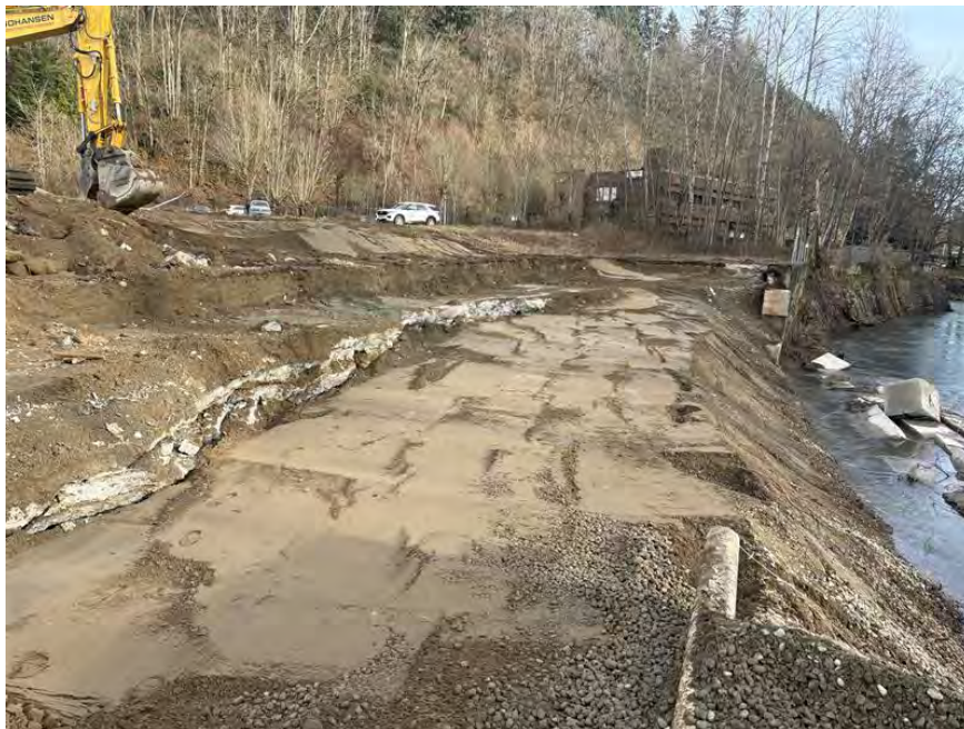
Pic 2. Exposed concrete bench above high-pH soils, looking east.
