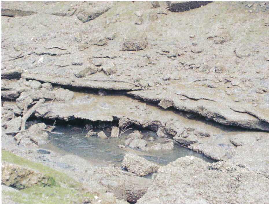
Waste Concrete Flows - North Bank - East Side of Neck (view to north)
