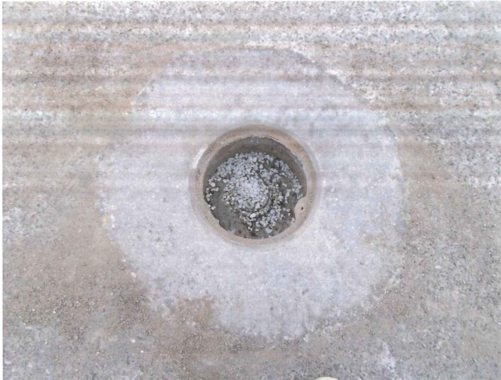
PHOTO NO. 1: Monitoring well MW-11, casing is filled with bentonite.
