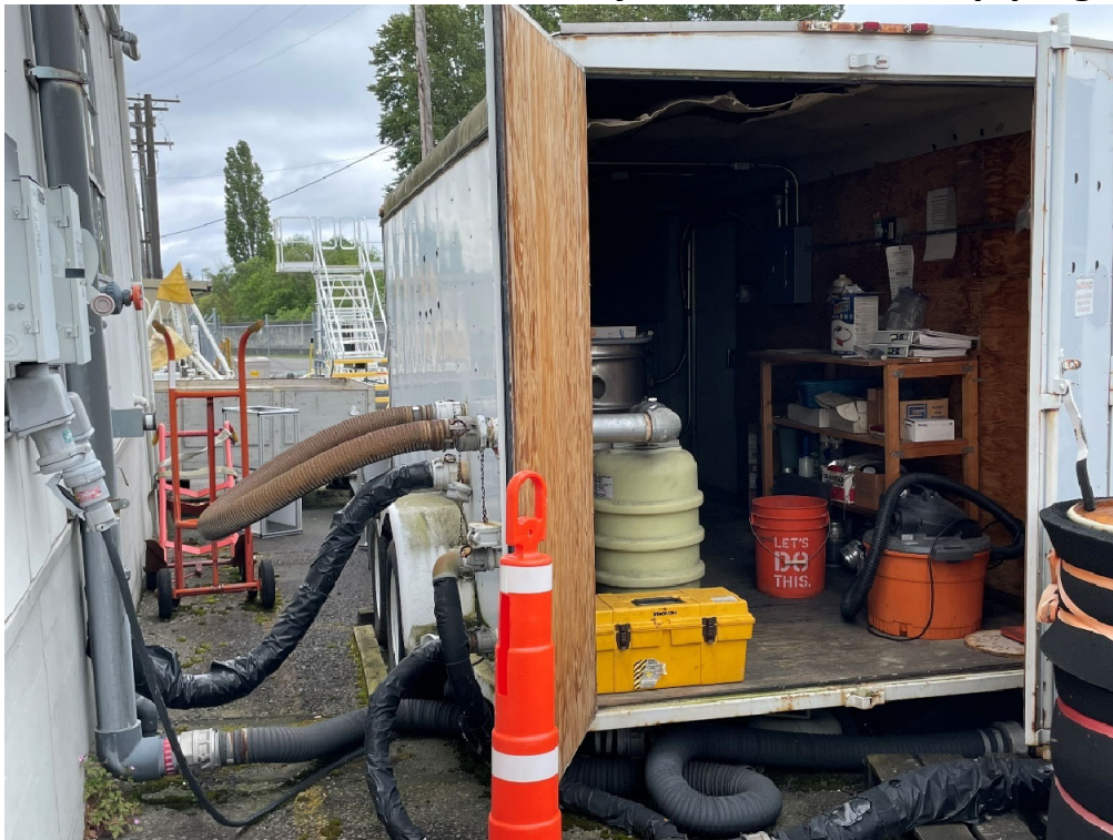
Photo 6: SWMU-172/174 SVE system trailer with piping shown.
