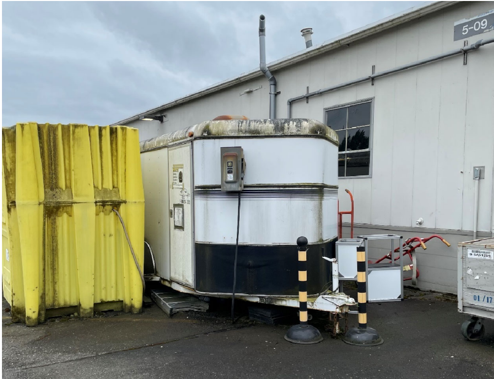
Photo 5: SWMU-172/174 SVE system trailer, adjacent to Building 5-09.
