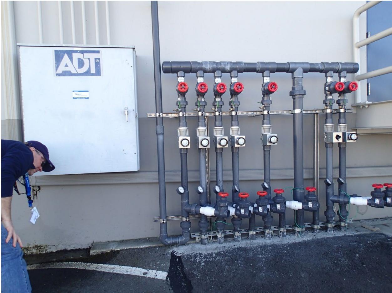
Figure 1: An Ecology inspector examines Boeing Renton's vapor intrusion mitigation system.
