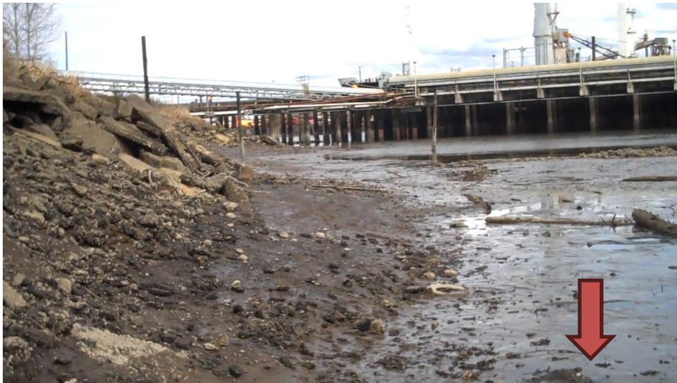
Photo 3: Deep seep location within the Embayment
