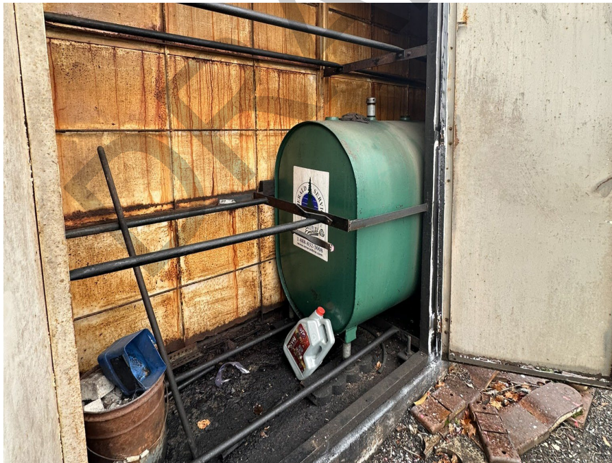
Photo 2. Aboveground waste oil tank in exterior cabinet north of the building.
