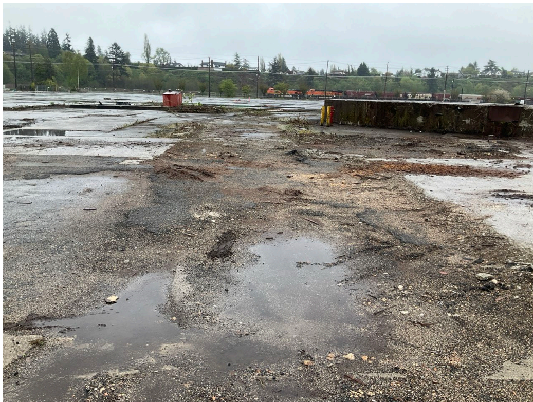
Photograph 6. Polygon B4 with broken concrete/asphalt between slabs.
