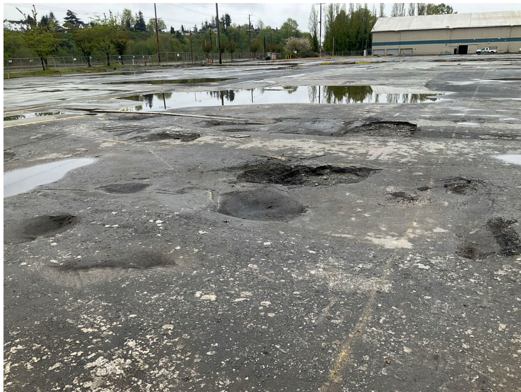
Photograph 8. Polygon B7 showing small areas of broken asphalt.
