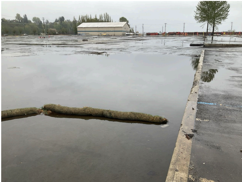
Photograph 22. Polygon F3: ponding near Outfall 4.
