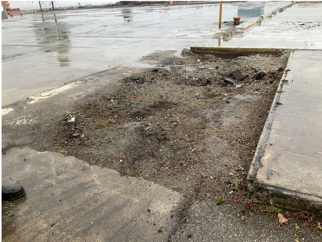
Photograph 5. Polygon B1 with broken asphalt and debris.
