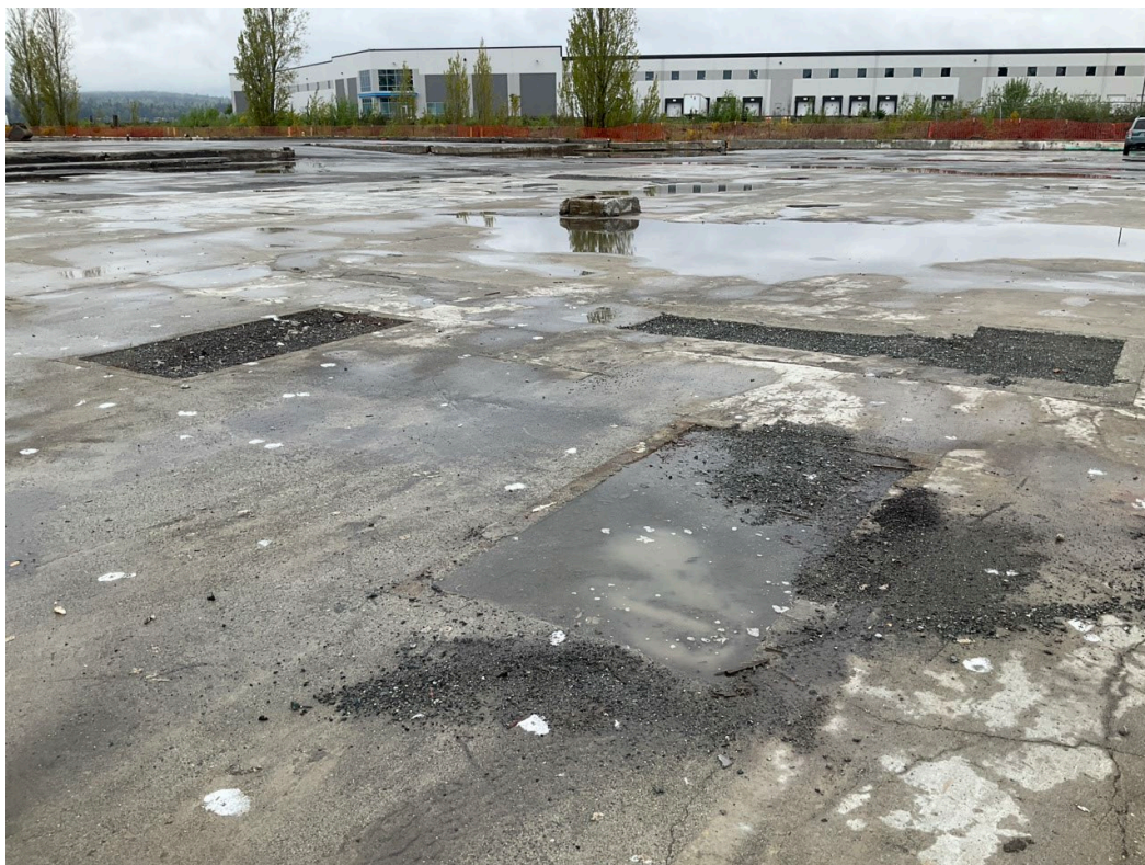
Photograph 7. Polygon B6 showing gaps in concrete with fill.
