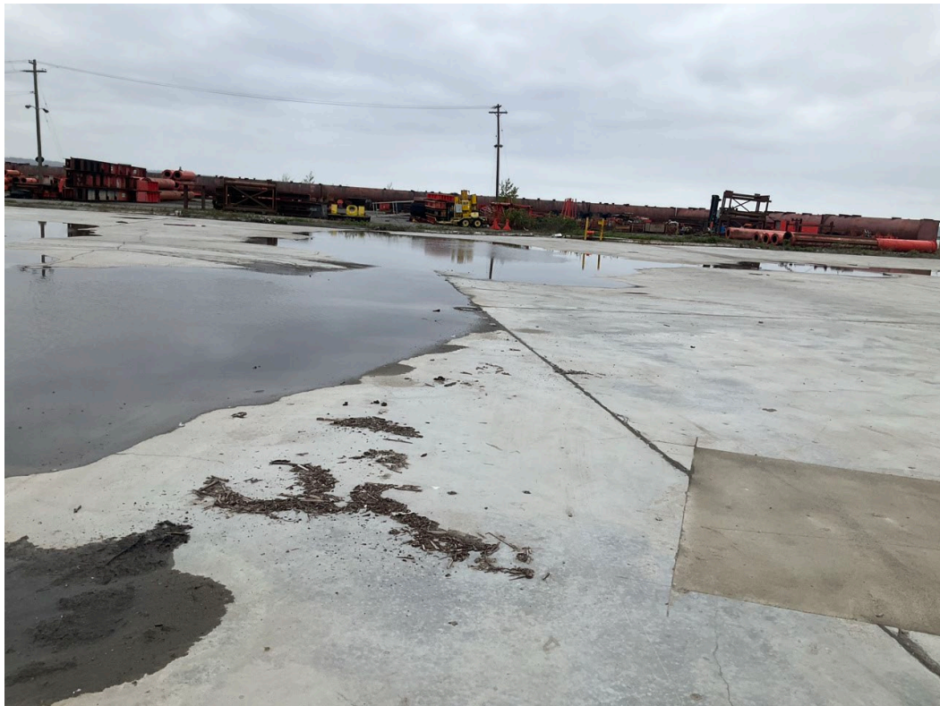
Photograph 25. Polygon F16: ponding over intact concrete.
