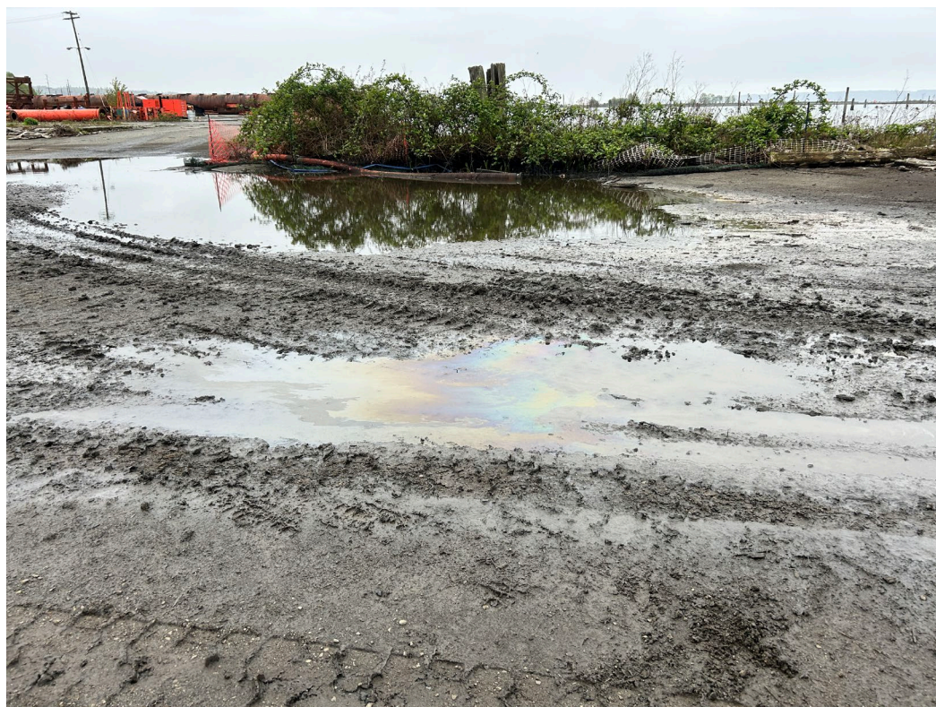
Photograph 24. Polygon F13: ponding near Outfall 5.
