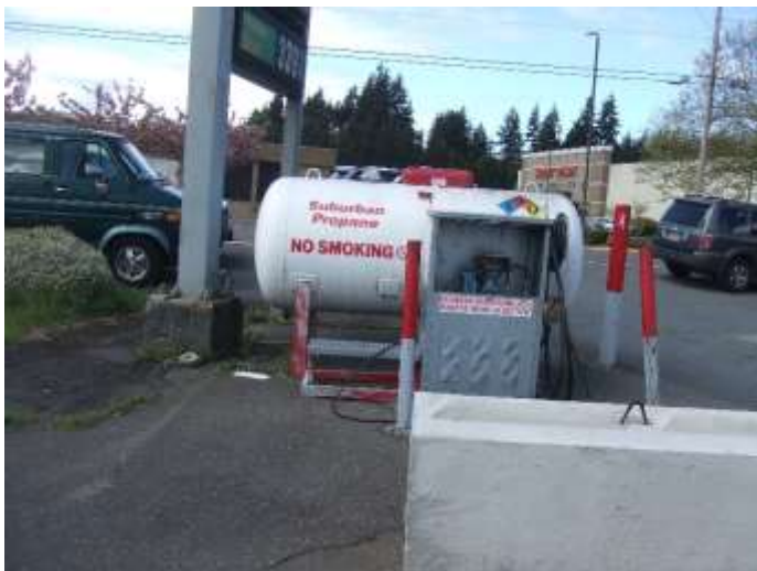
Photo 3. View of the propane tank.
