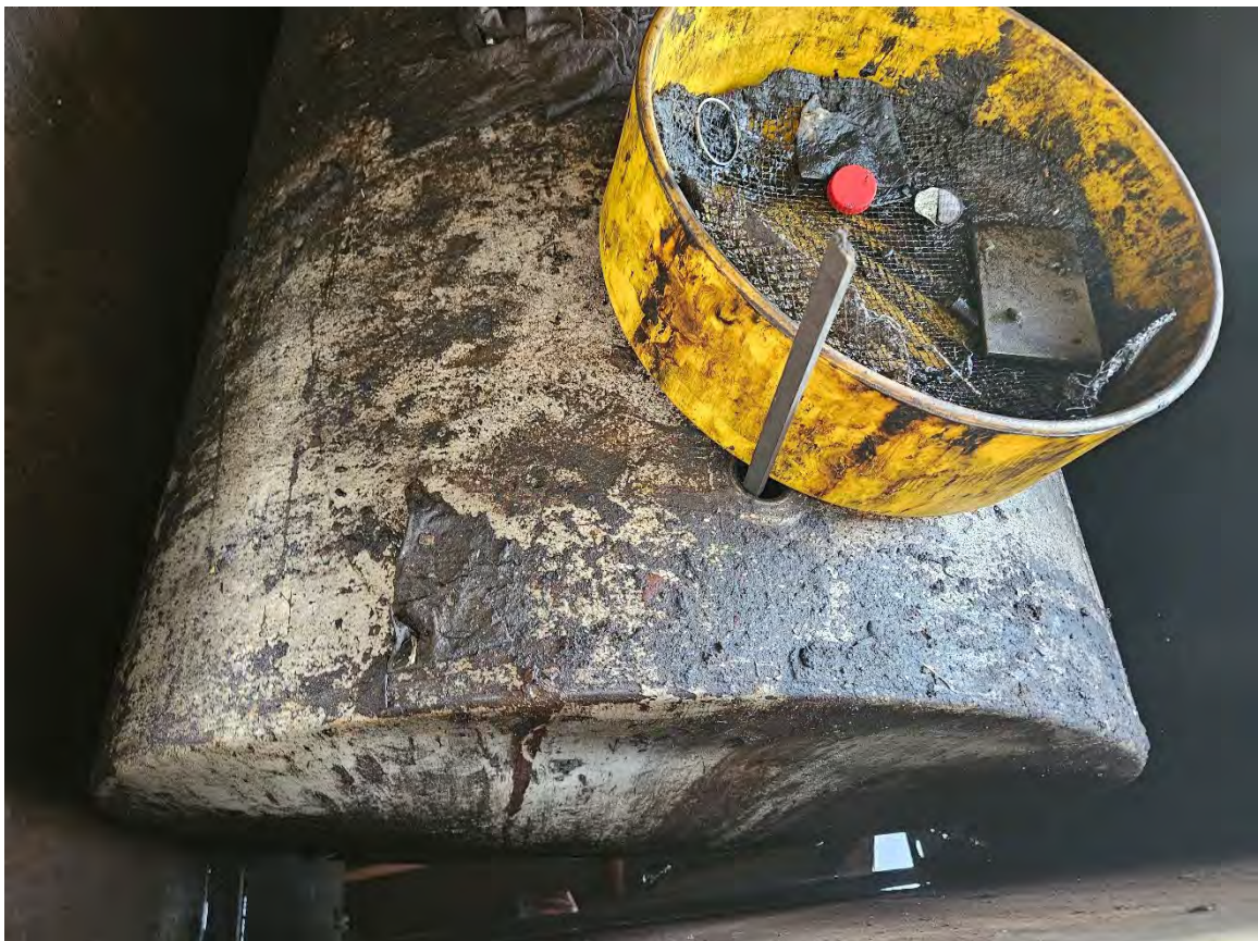
The storage tank inside the dumpster with an unknown fluid pooled in the bottom.
