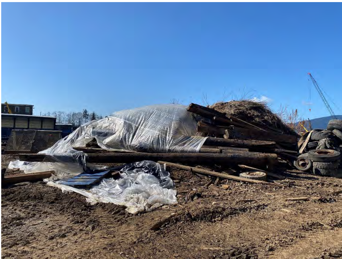
View of the soil stockpile. Note separated piles of creosote piles and tires.
