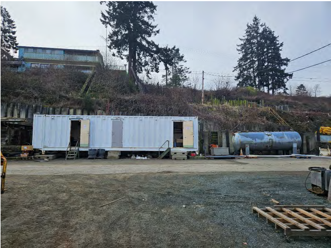
New office container with adjacent tank to be used for sewage storage.
