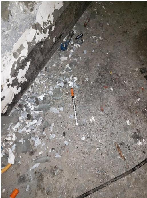
Photo 4: Hypodermic needle next to the TC-24 transformer. Taken from the 2 nd floor TC-24 Transformer room.
