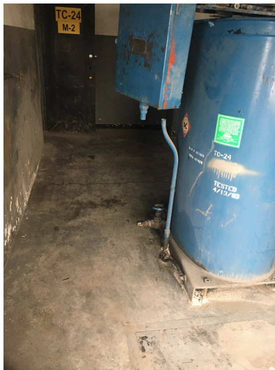
Photo 3: Transformer TC-24 Spill Area (second level) after to cleanup actions.
