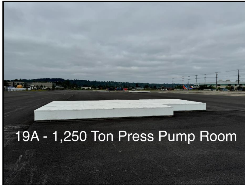
Photo 10, Facing West, 1,250 Press Pump Room Pit Cover
