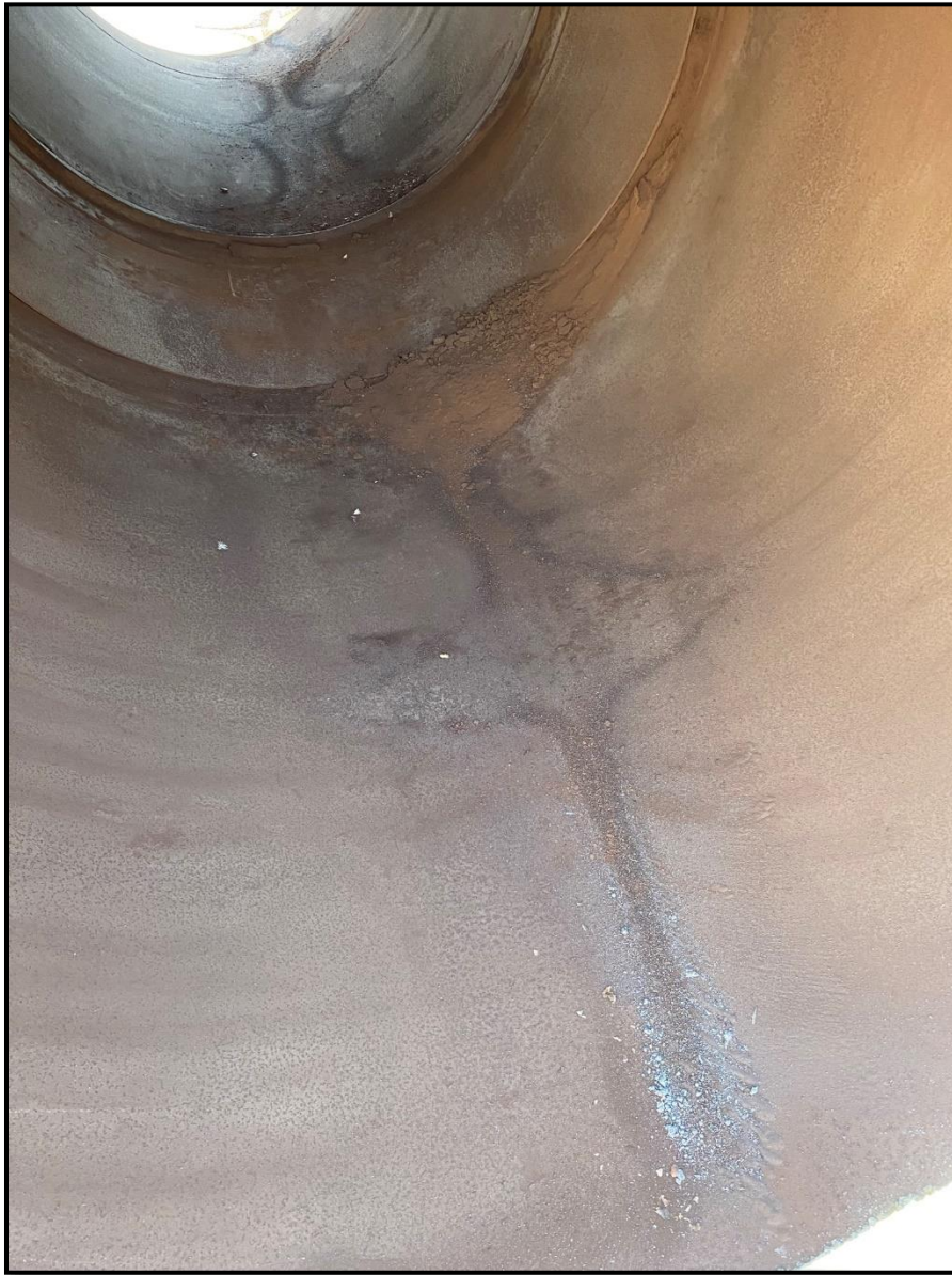
Photo BH-04: Example of Residual Baghouse Dust in the Duct Interior Requiring Removal Photo Taken: 9/21/2023
