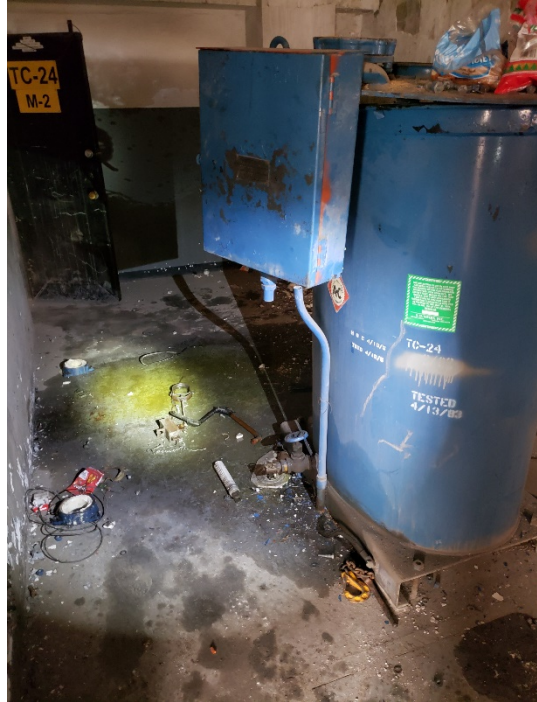
Photo 2: Transformer TC-24 Spill Area (second level) prior to cleanup actions.
