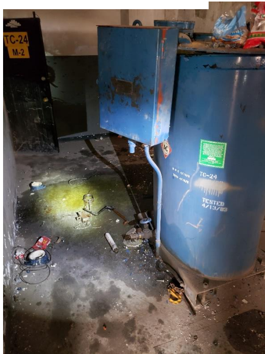
Photo 1: Transformer TC-24. Spilled oil visible on the floor. Taken from the 2 nd floor TC-24 Transformer room.
