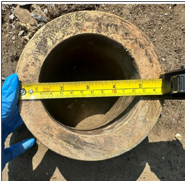
Figure 5-11. Finding of non diagnostic copper pipe in Central Accumulation Area/Oil Shed, facing plan
