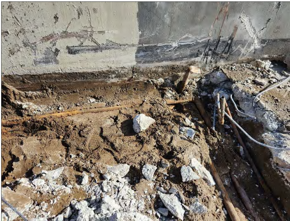
Photo 20: South Tank Vault, product line running from left to right (north to south), where it joins two other lines that used to stub up through the concrete slab floor. Those lines appeared to have been cut and bent at some point in the past. View to the east.
