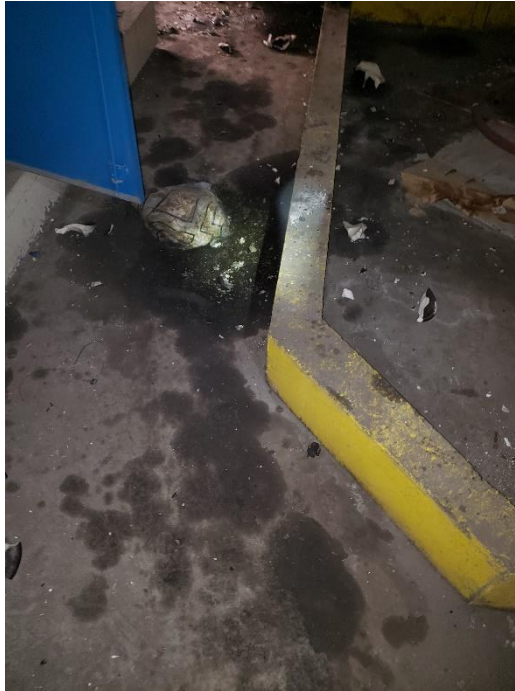
Photo 5: Spilled oil on the first floor beneath the TC-24 transformer room. Oil had dripped through the ceiling due to holes in the upstairs floor. Footprints are visible in the oil in the foreground.
