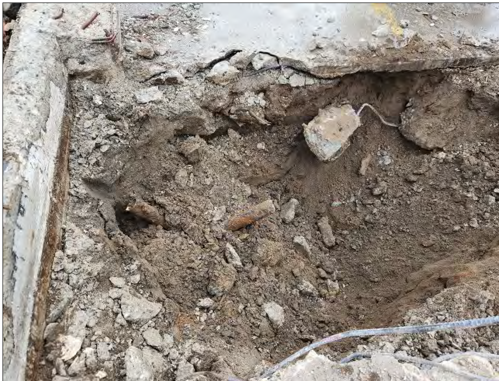
Photo 8: North Tank Vault, southernmost end of the product piping. The piping had been cut just inside the foundation wall of the aluminum building. A cap was still present on the end of the pipe.
