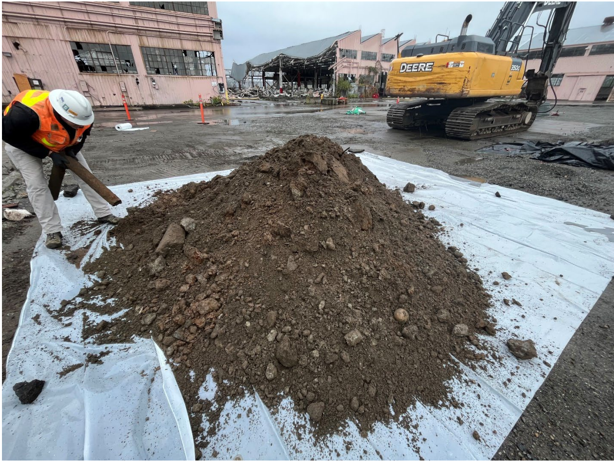
Figure 2. Soil removed from under foundation near the northern wall of the Aluminum building.
