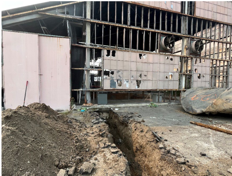
Figure 4. Unidentified piping running out of North Vault with Aluminum Building.
