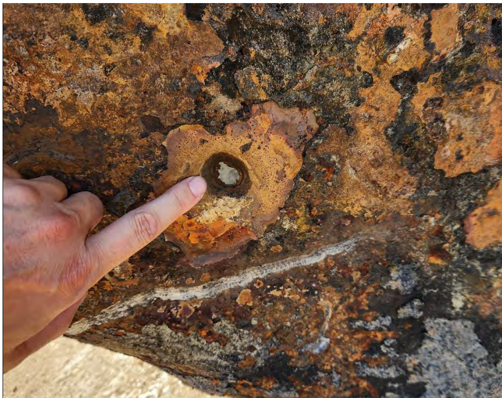
Photo 16: South Tank Vault, example of a pinhole caused by corrosion. These were visible on multiple tanks.
