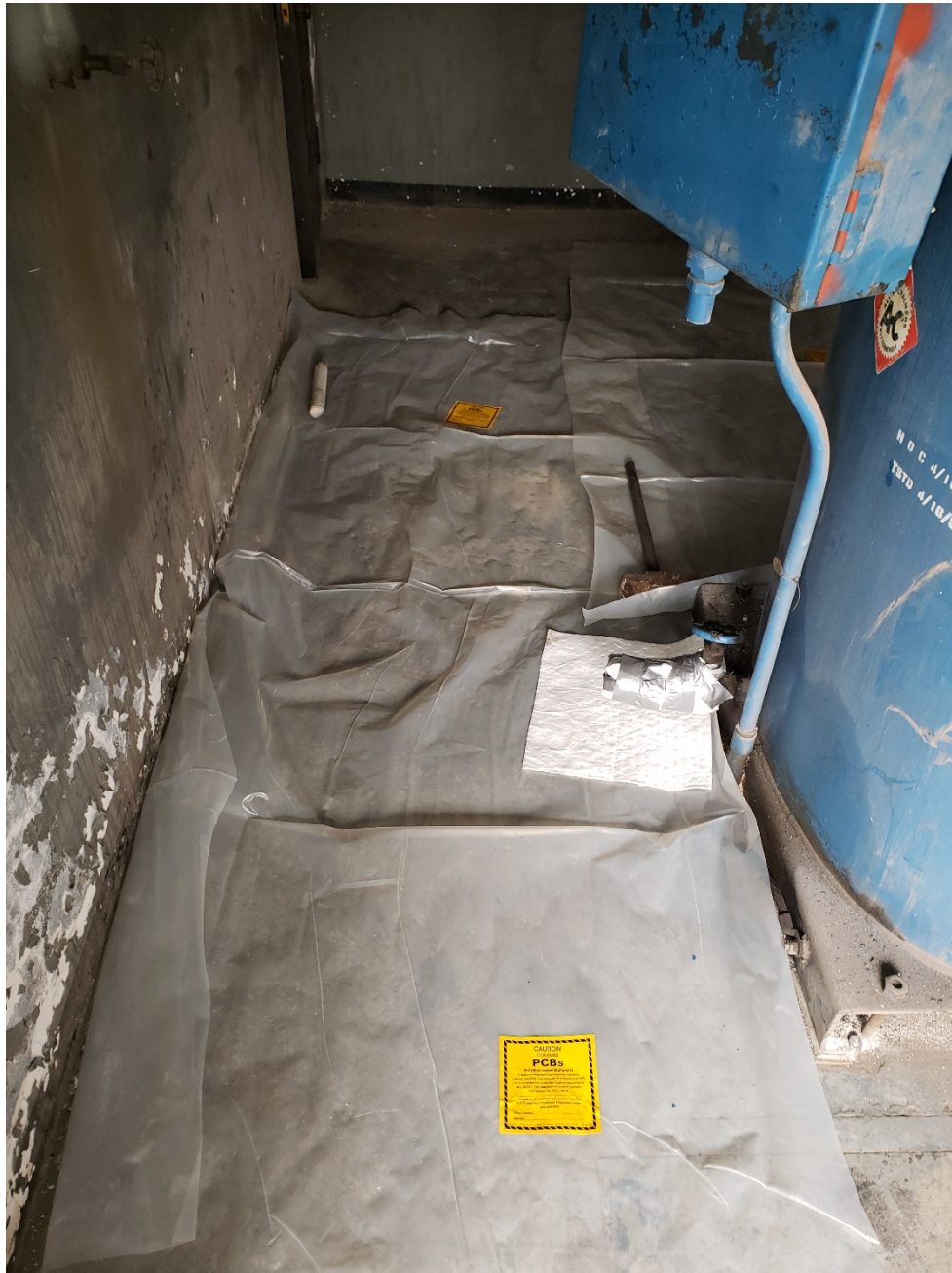
Photo 4: Transformer TC-24 Spill Area (second level) after to cleanup actions. The drain valve was damaged but has now been secured. A spill pad has been placed on the ground to capture any drips and visqueen was placed on the ground of the impacted area.
