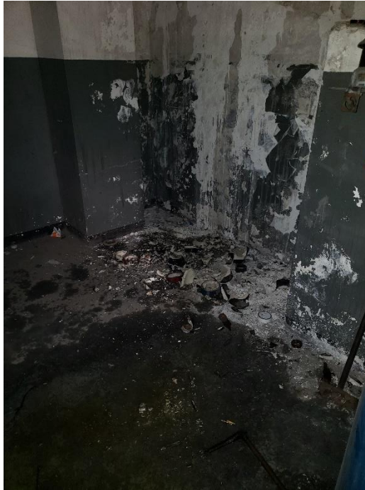
Photo 3: PCB oil on the floor behind transformer TC-24. Broken ceramic insulators and debris also visible. A hypodermic needle is visible in the background. Taken from the 2nd floor TC-24 Transformer room.
