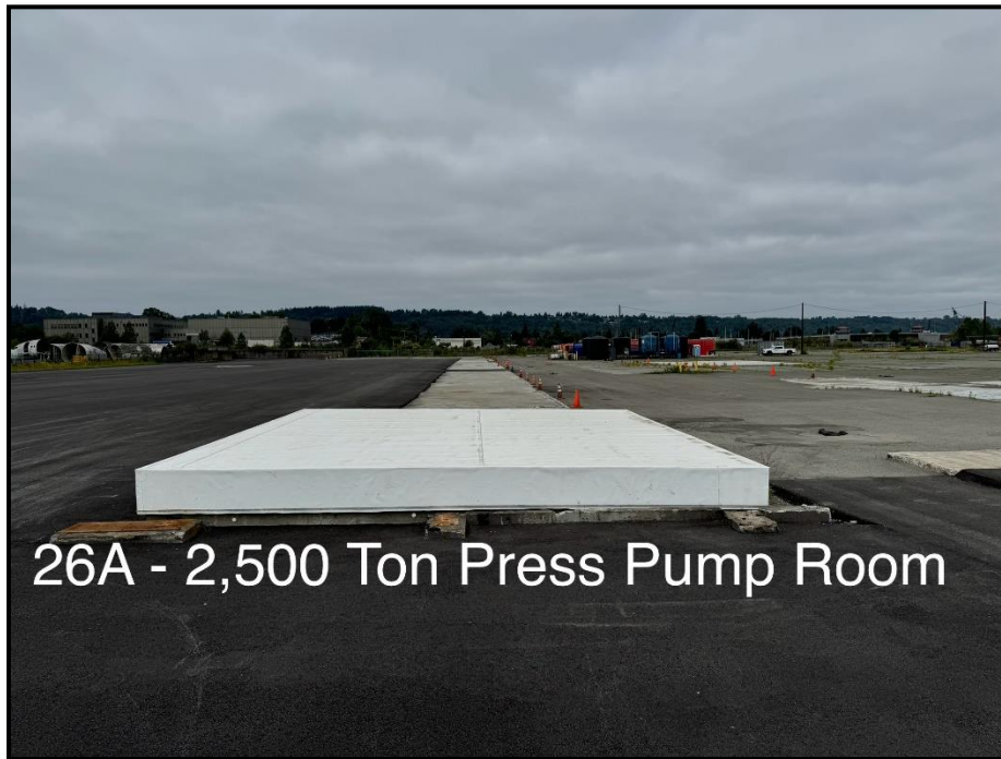
Photo 07, Facing West, 2,500 Ton Press Pit Pump Room Pit Cover
