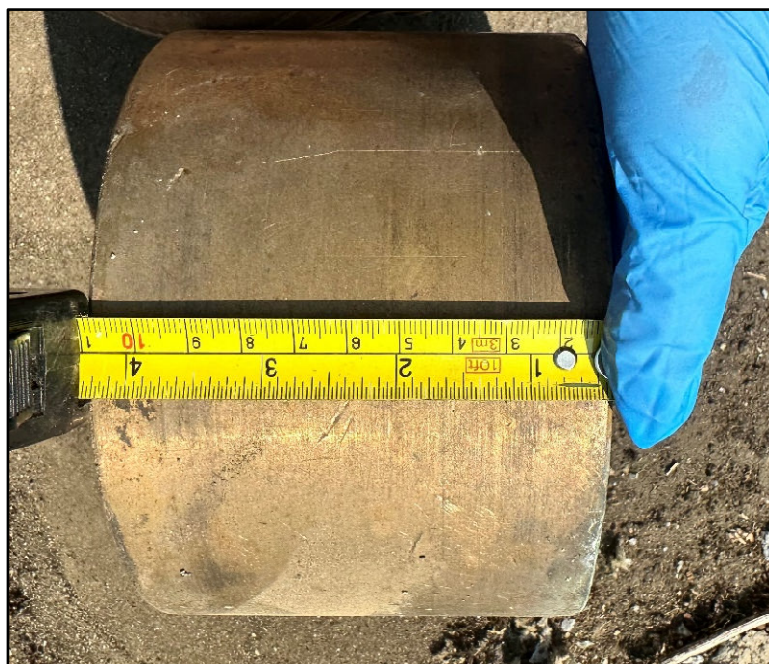
Figure 5-12. Finding of non-diagnostic copper pipe in Central Accumulation Area/Oil Shed, facing plan
