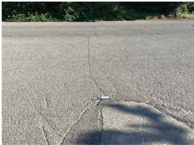
Photo 10: Terminal 115 Driveway - Transverse Cracking.
