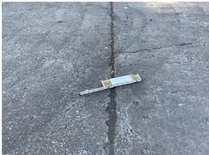
Photo 14: Former Unimacts Global, LLC Lease Area - Concrete Joint.
