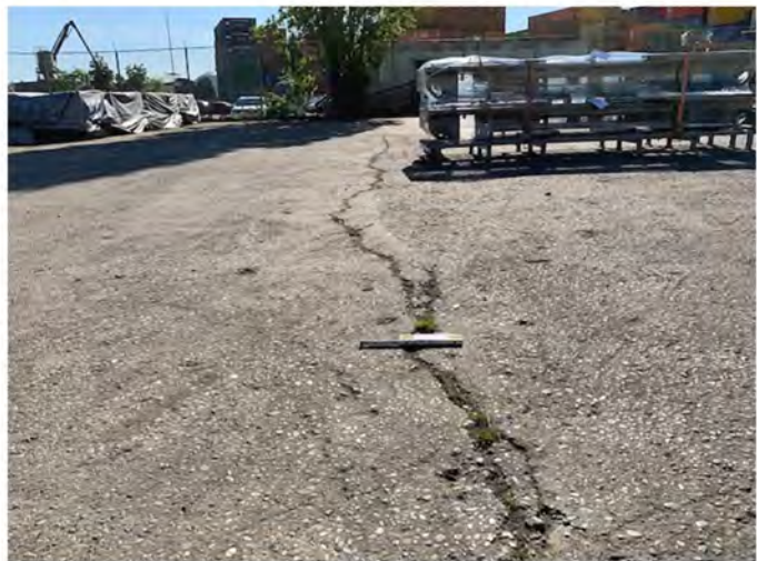
Photo 15: Former Unimacts Global, LLC Lease Area - Cracks in Concrete Surface.
