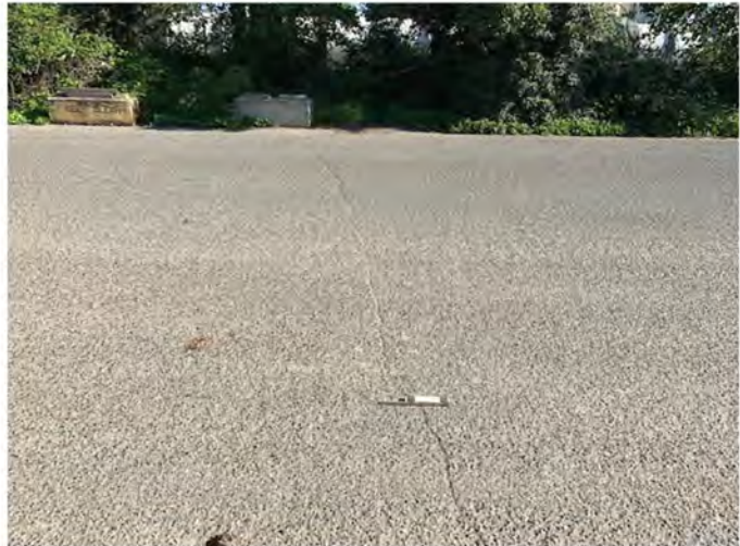
Photo 11: Terminal 115 Driveway - Transverse Cracking.
