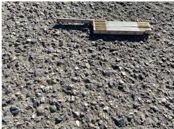
Photo 13: Former Unimacts Global, LLC Lease Area - Concrete Surface Wear.
