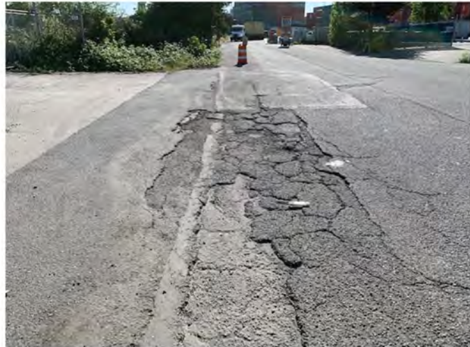
Photo 12: Terminal 115 Driveway - Spider Web Cracking.
