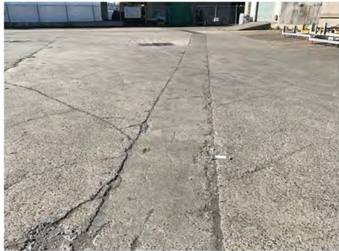
Photo 16: Former Unimacts Global, LLC Stormwater Drain Line Patch.
