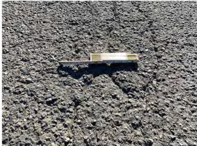
Photo 9: Terminal 115 Driveway - Asphalt Surface Wear.
