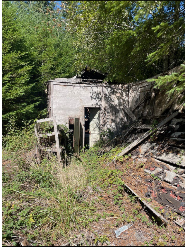
Photograph B-7. Building 1864 Former Fire Station foundation and debris
