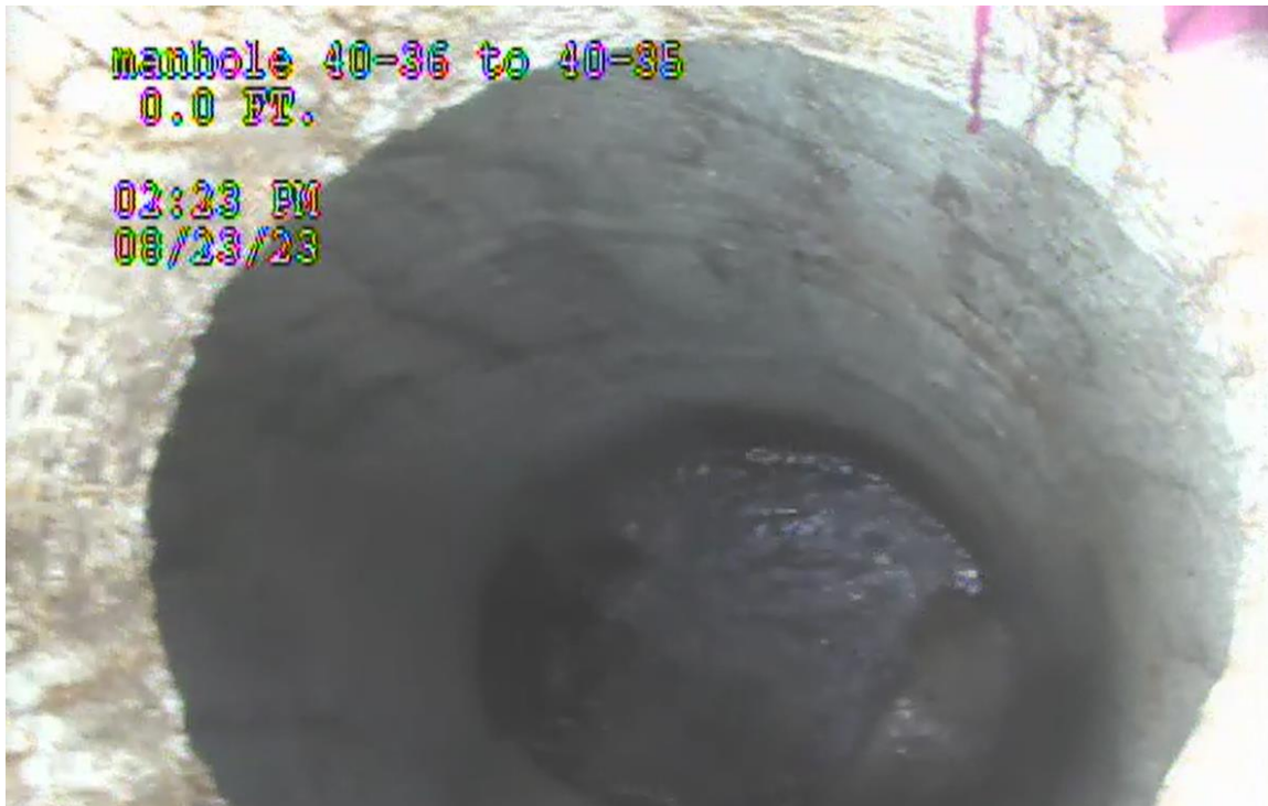
Figure 2: MH 40-36 showing approximately 6" of water in the bottom of the manhole.
