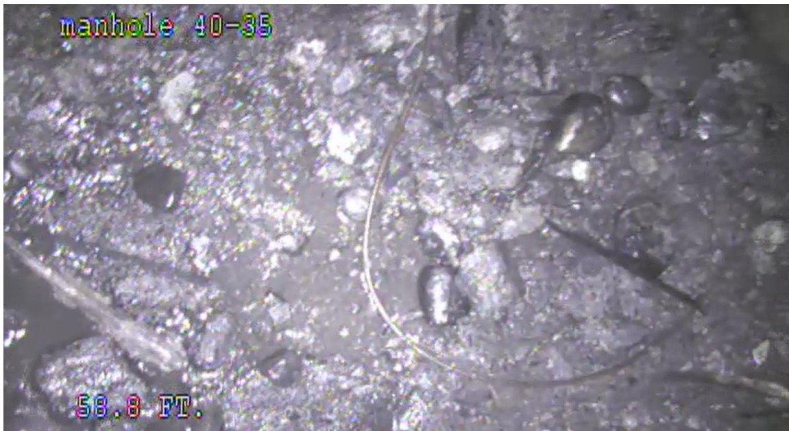
Figure 1: Video still from MH 40-35 showing rocky debris and cable lifting loops.
