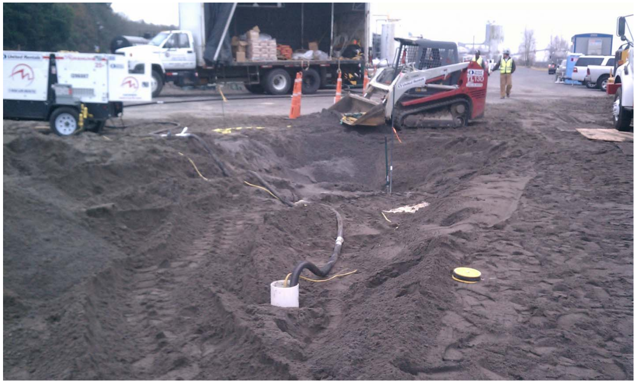
Photograph 13: Extraction well pumping.
