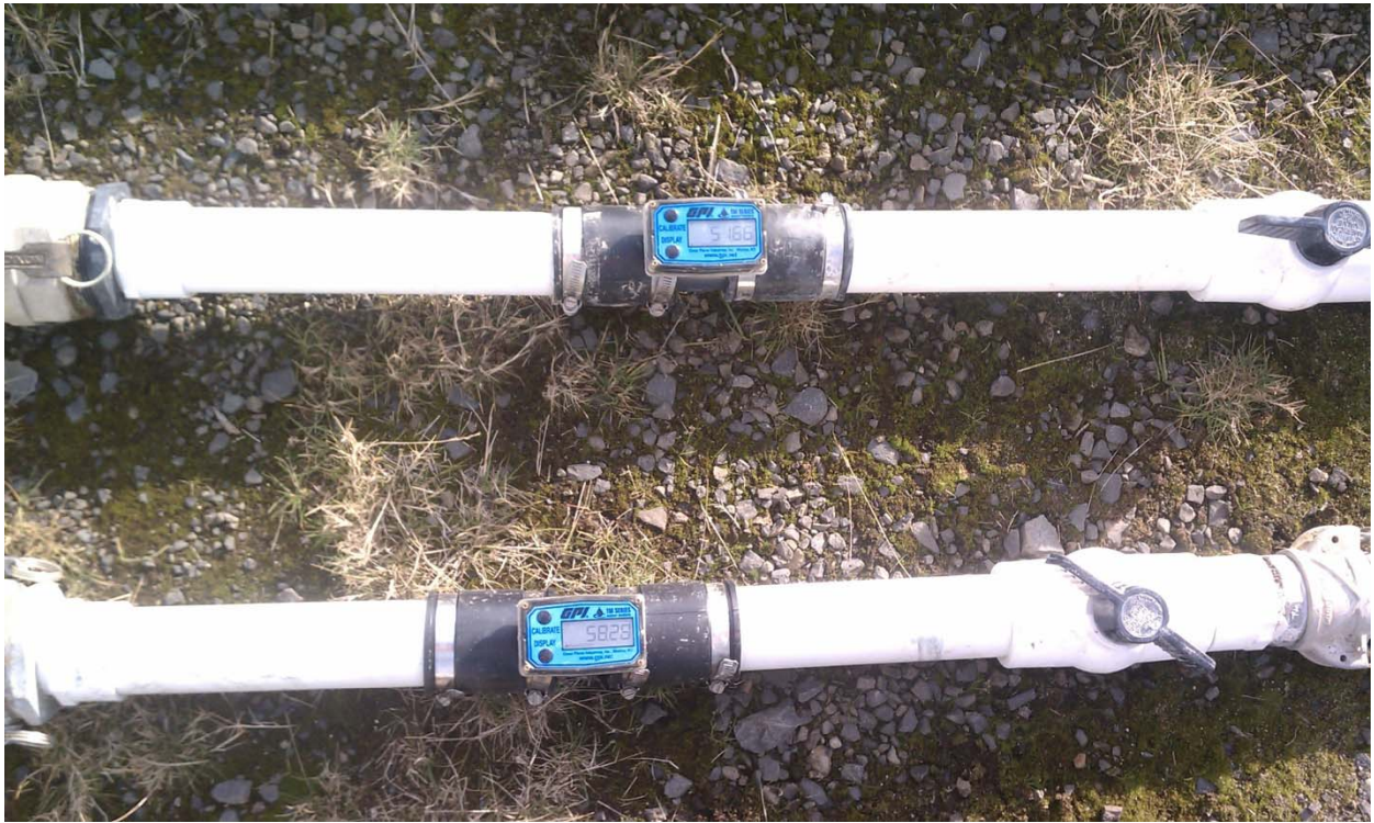
Photograph 17: Totalizing flow meters and flow control valves in two legs off injection manifold.
