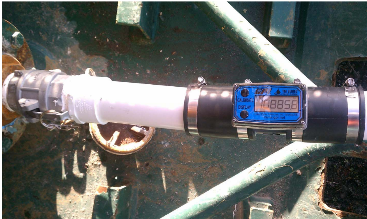
Photograph 18: Totalizing flow meter.
